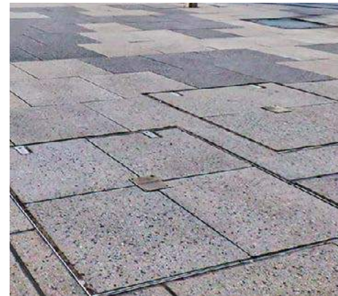
Discrete utility access cover
