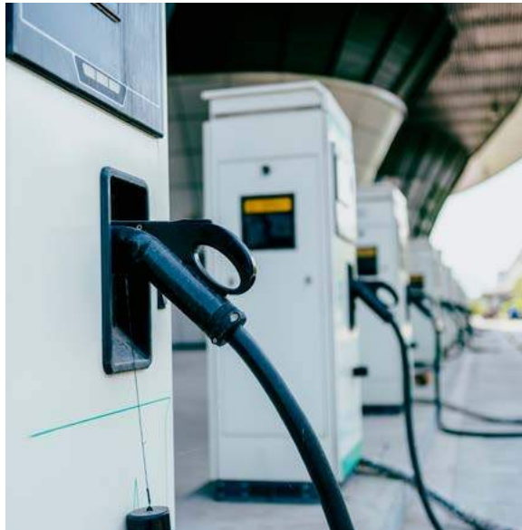
Electric Vehicle Charging Stations
