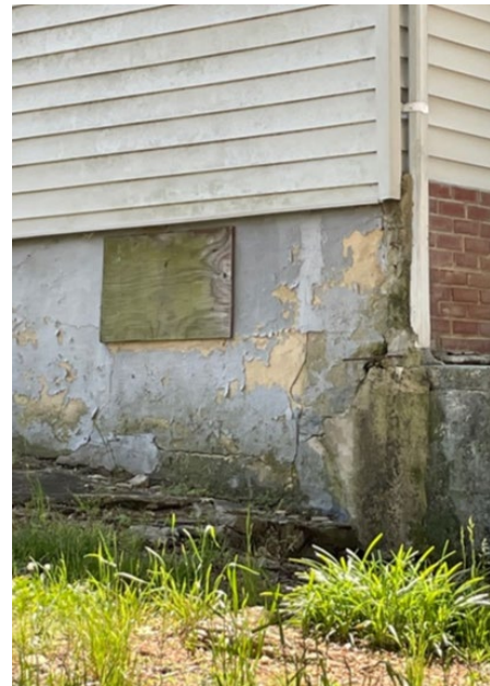
4. Pressure Bulge on foundation 2022
