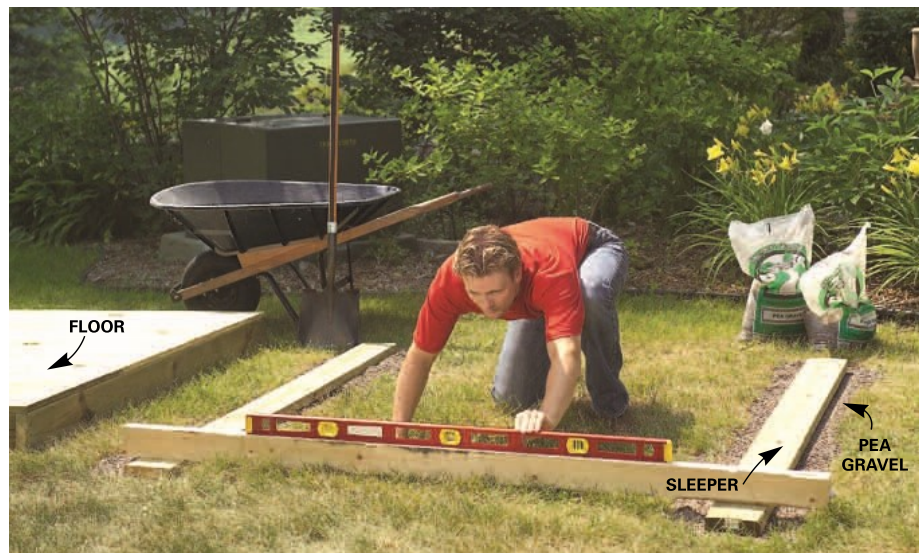
5 Dig two trenches 6 in. deep and fill them with pea gravel. Then level treated 2x6 sleepers over the gravel and set the floor on the sleepers.
