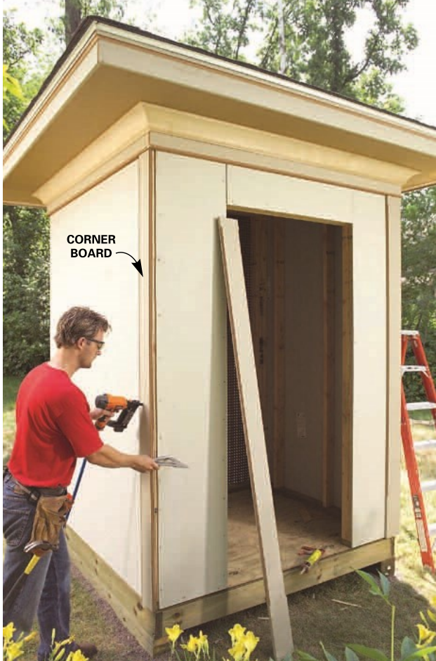
10 Nail and glue the corner boards in place. Install the narrower side first, making sure it's flush with the corner. Then add the full-width piece.
