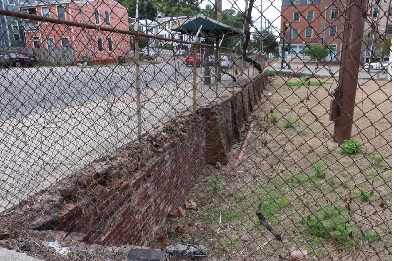
7. Grade drop between sidewalk and property.
