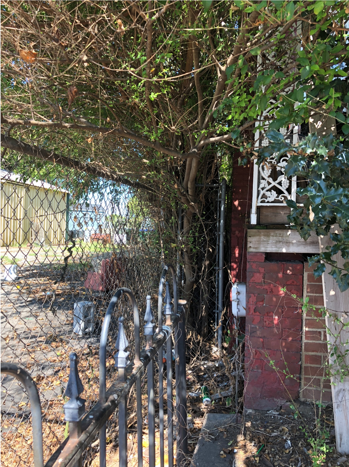
Image 3 – Overgrown trees and vines are present at the perimeter of the lot along the chain link fence.
