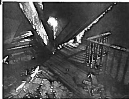
Figure 8: Water damage and bearing failure of roof valley beam
