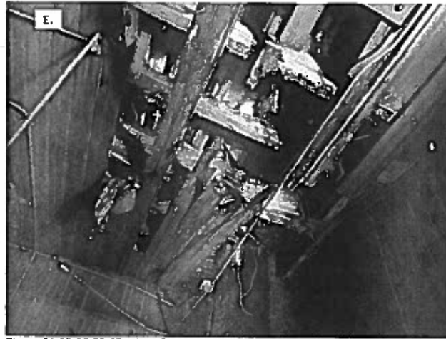
Figure 9A,9B,9C,9D,9E. Water Damage on Lower Levels Due to Roof Valley Beam Failure
