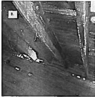
Figure 14: Poor Bearing on 3rd Floor Rear Wall
