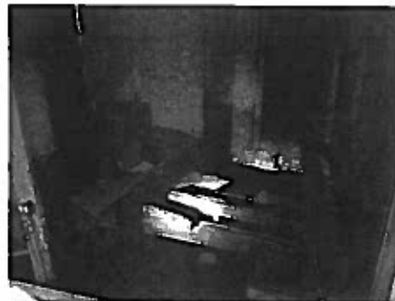
Figure 18: Damaged and missing 1st floor framing
