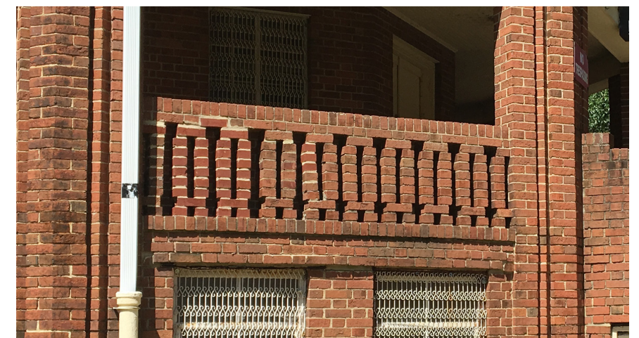
DAMAGED EXISTING BRICK RAILINGS
