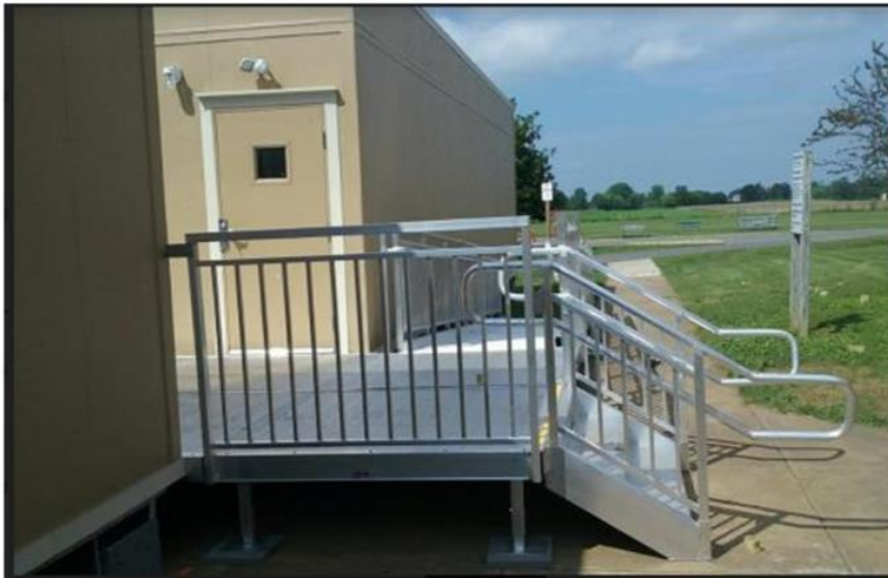
Figure 3 Typical Metal Ramp/Stair Combination
