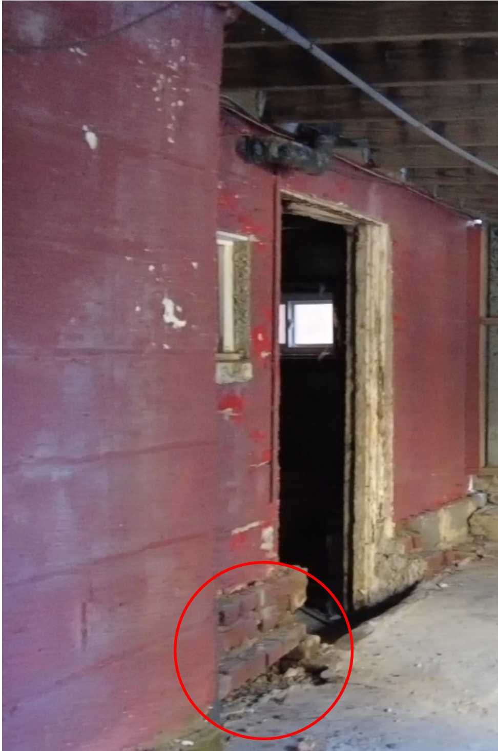
Photo above showing the brick footing in declining condition.
