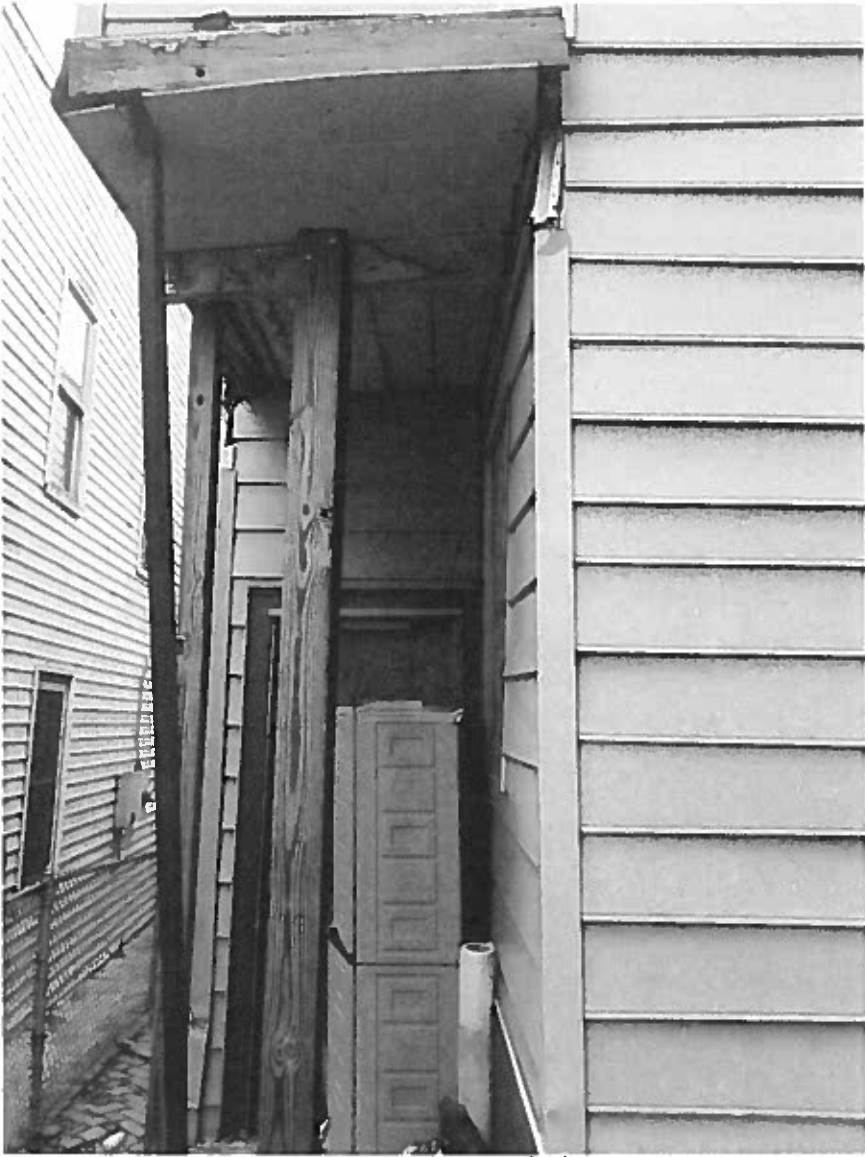
- Back left of Structure (Lower) (improve continuity & structure).
