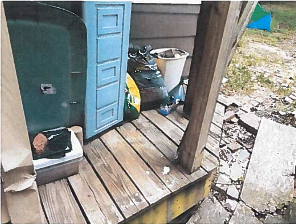
- Back Porch Area (supports to be brought to code).
