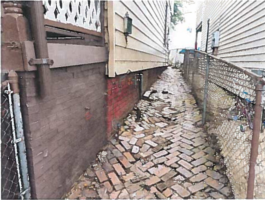
- Distressed Brick Walkway and Fence (replace bricks with concrete and privacy fence.)
