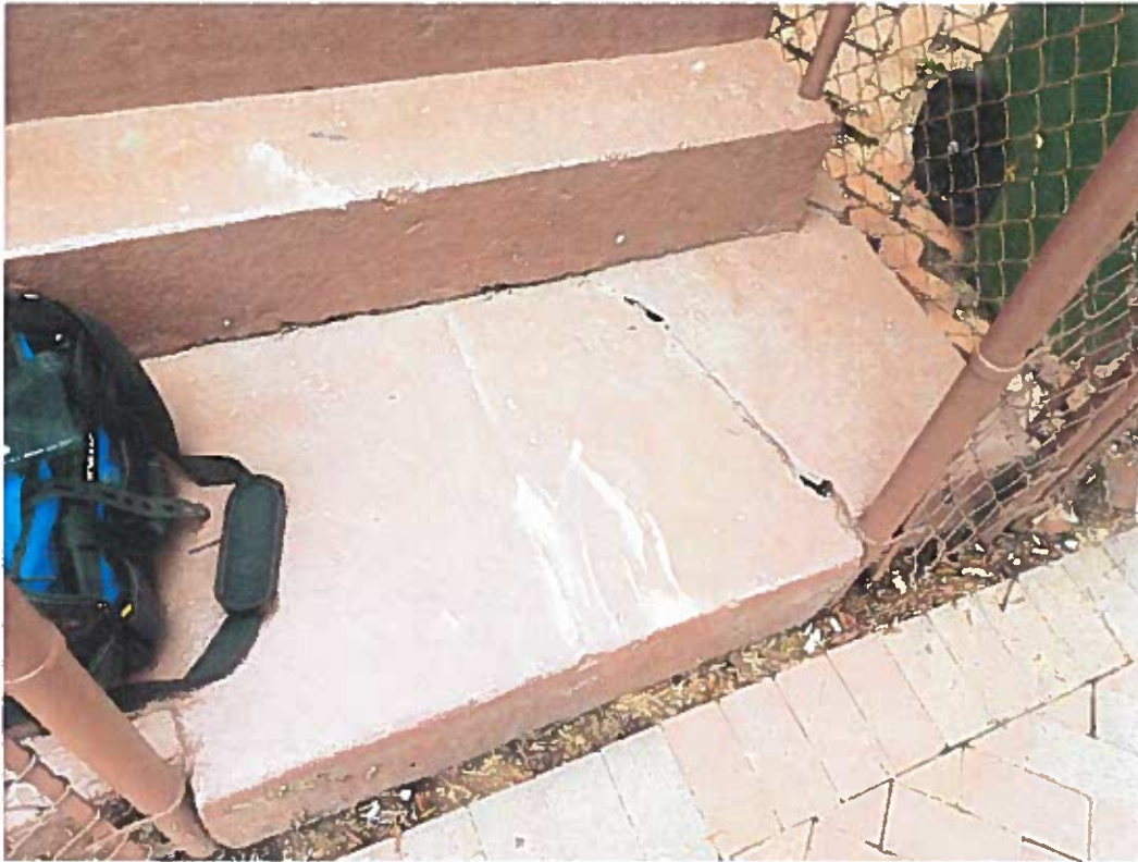
-Front Steps (Cracked concrete, to be demo'd and brought to code.
