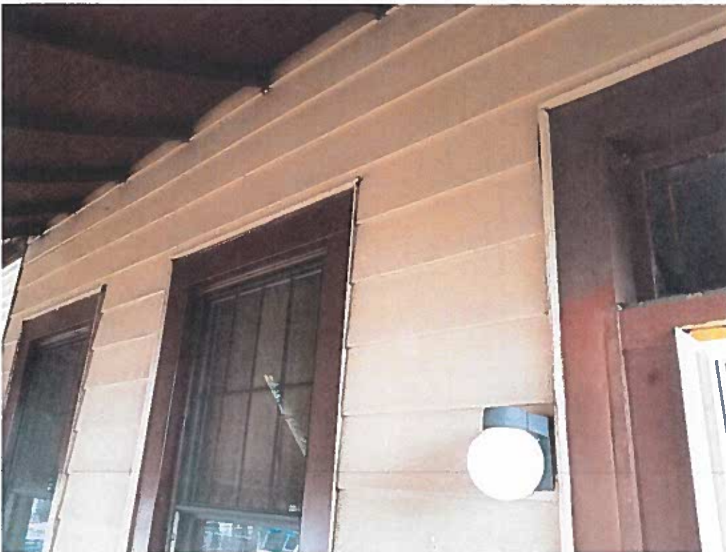
-Porch Ceiling and Siding (porch ceiling to be painted and siding replaced.
