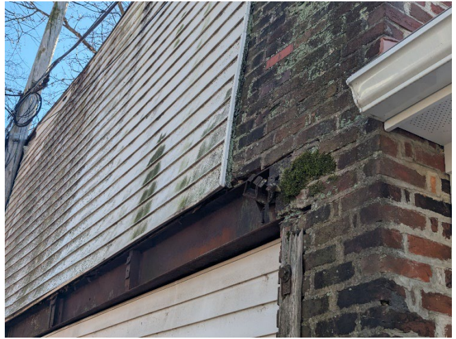
Figure 7: deterioration of the historic brick
