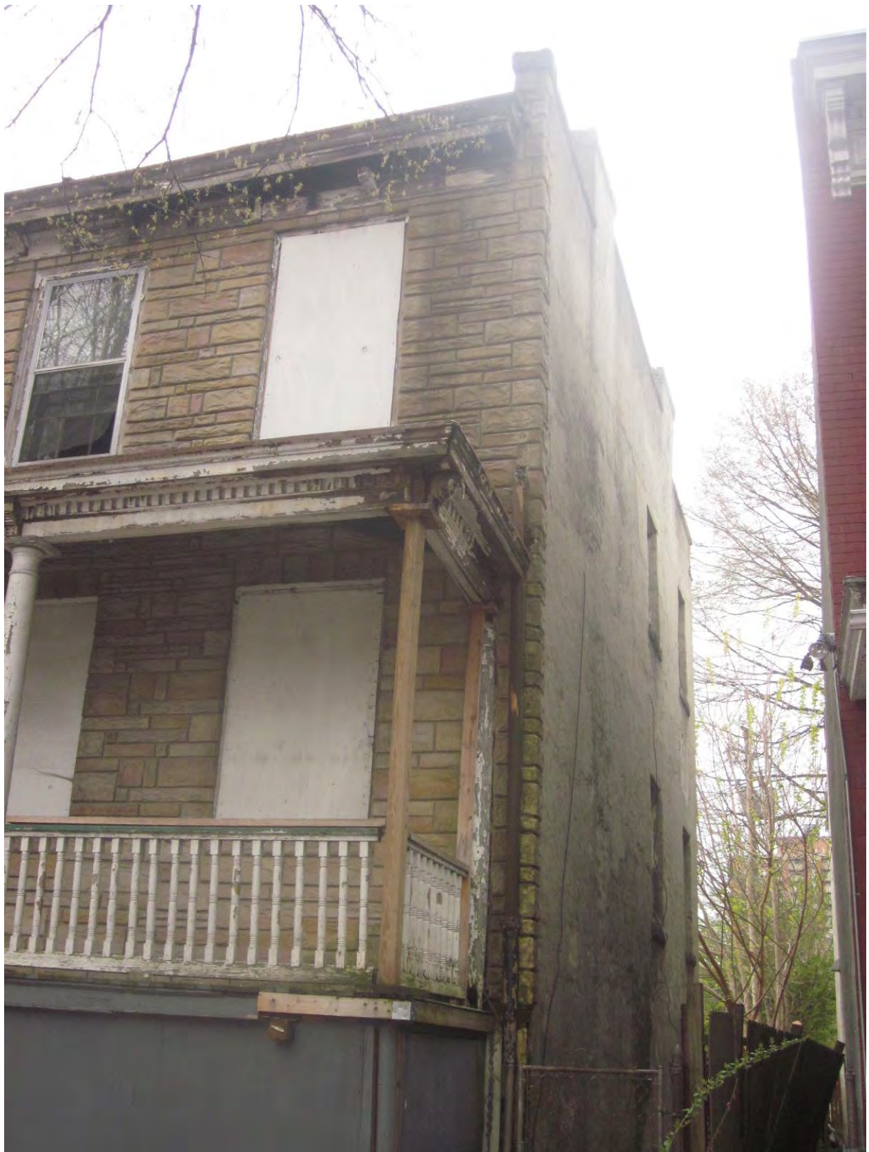
511 West Marshall Street, Richmond, VA Part 2 Photos; DHR #2018-070; NPS Proj. # Not Yet Assigned Photo 2.1 Gutters and Downspouts; Exterior Walls/Masonry
