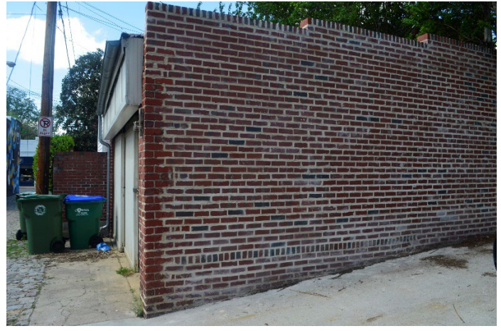
Figure 6. Existing brick veneer wall on the east side which was built sometime after 2011.
