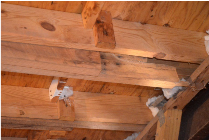
Figure 7. Interior view of the structurally unsound roof in the garage.
