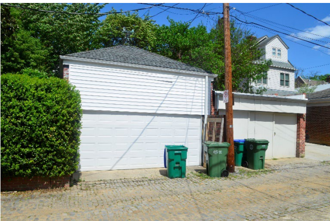
Figure 15. 2917 Monument Avenue garage. The façade of this garage appears to have been modified at some point. The 2915 Monument Avenue garage can be seen on the right side of the photograph.
