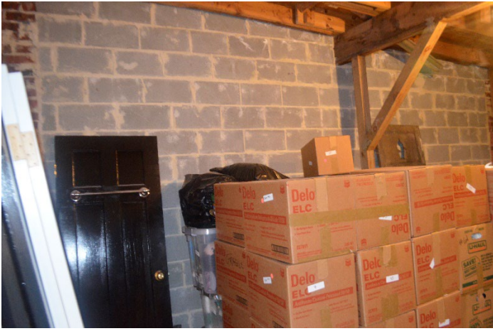
Figure 5. Interior view of the garage's replaced east wall, which was built sometime after 2011.
