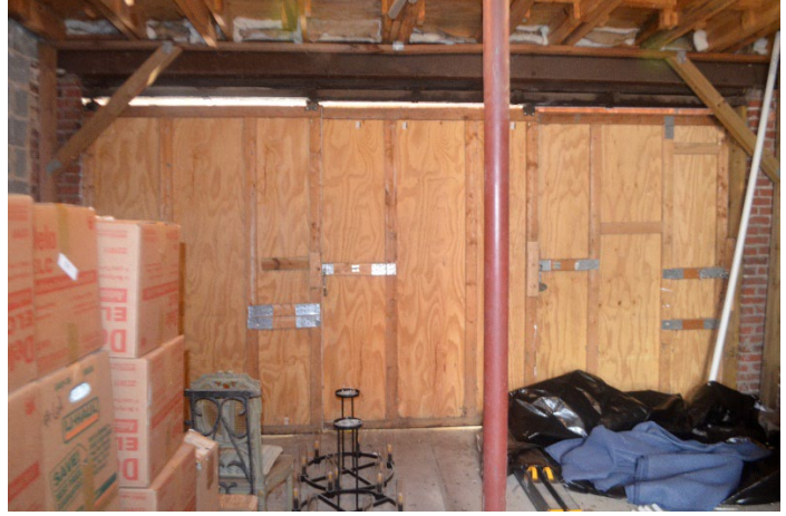
Figure 2. Interior of the garage door which will be replaced with a new, automatic door.
