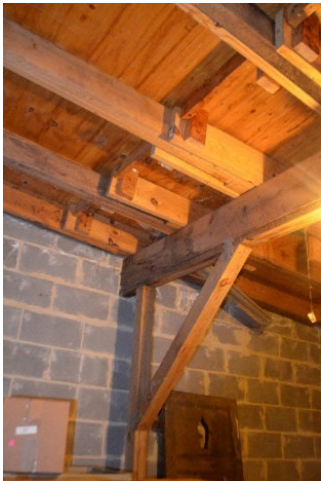
Figure 9. Interior view of the garage's east wall. The photograph shows additional wall braces added to support the unsound roof.
