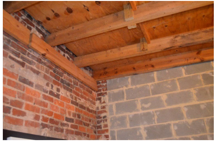
Figure 8. Interior of the garage showing the northeast corner, and the replacement east wall.
