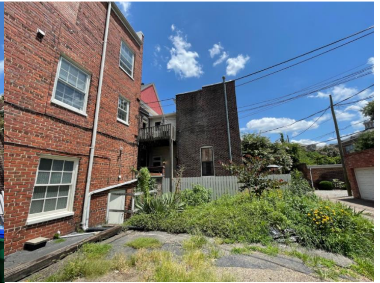
Figure 6. View of existing 2 nd story deck and location of proposed rooftop deck from the alley
