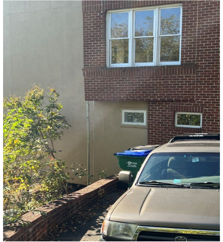
Figure 2. areas in need of repair
