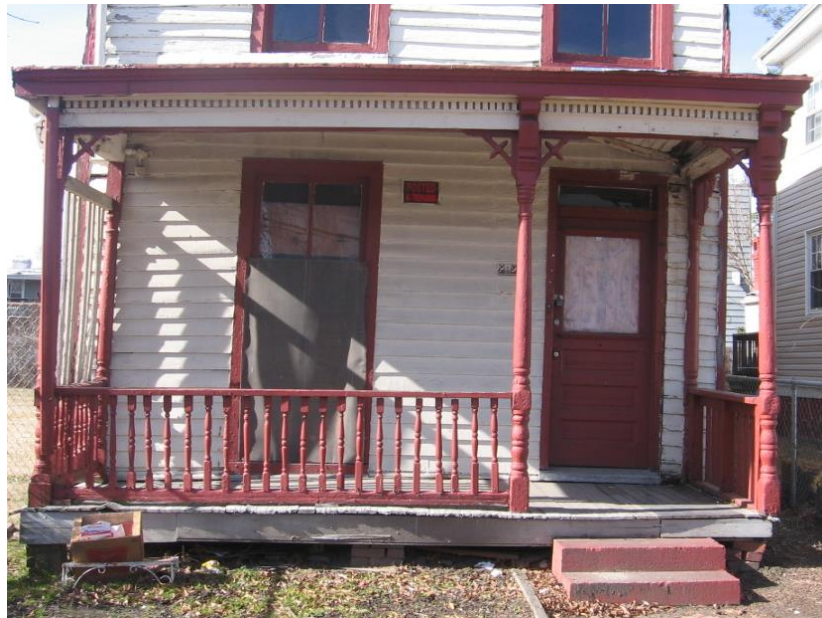
818 North 25 th Street Railing (February 2015)
