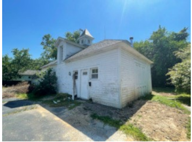
Figure 2. 4002 Existing Rear Carriage House, 2021. Hipped roof with through-the-eave dormer and cupola. (pre-rehabilitation).
