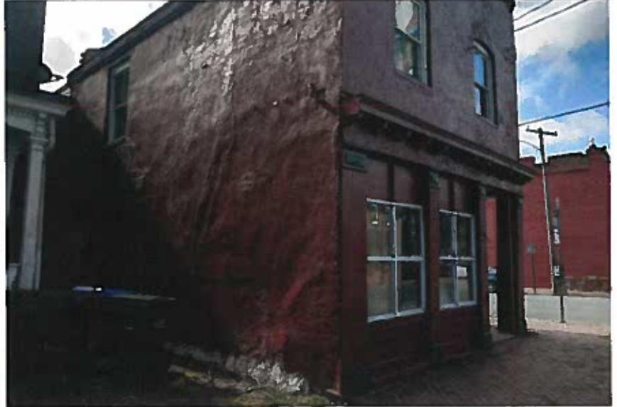
CURRENT CONDITIONS: NORTH AND WEST FACADES REPAIR STUCCO AND DENTIL MOULDING AS REQUIRED. PAINT STUCCO, WOOD TRIMWORK IN ACCORDANCE WITH CAR GUIDELINES. ADD OPENING TO NORTH WALL TO ACCOMODATE DUCT FROM COMMERCIAL GAS RANGE AND GRILL.
