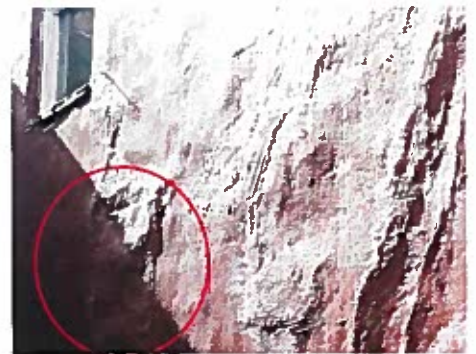
CURRENT CONDITIONS: NORTH FACADE PRE-EXISTING PATCHED OPENING TO BE REOPENED FOR RANGE HOOD OUTLET
