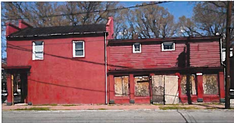
CURRENT CONDITIONS: SOUTH FACADE REMOVE BOARDS AND REPAIR/REPLACE WINDOWS AND DOORS TO MATCH HISTORIC PHOTOS, PAINT STUCCO, WOOD SIDING, AND TRIMWORK IN ACCORDANCE WITH CAR GUIDELINES
