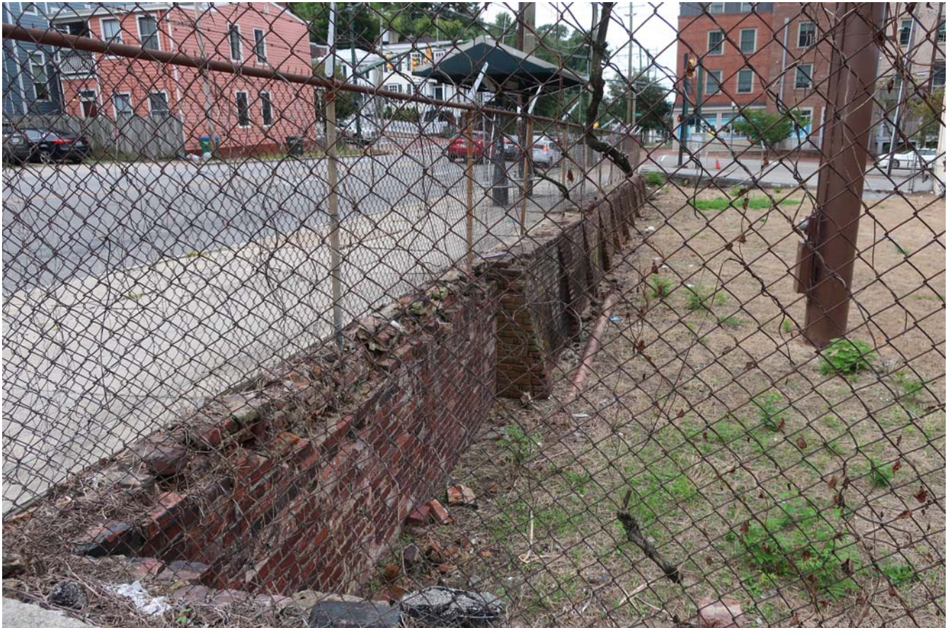
7. Grade drop between sidewalk and property.
