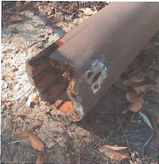
#5 bottom of left corner column *this was the only intact column from the porch
