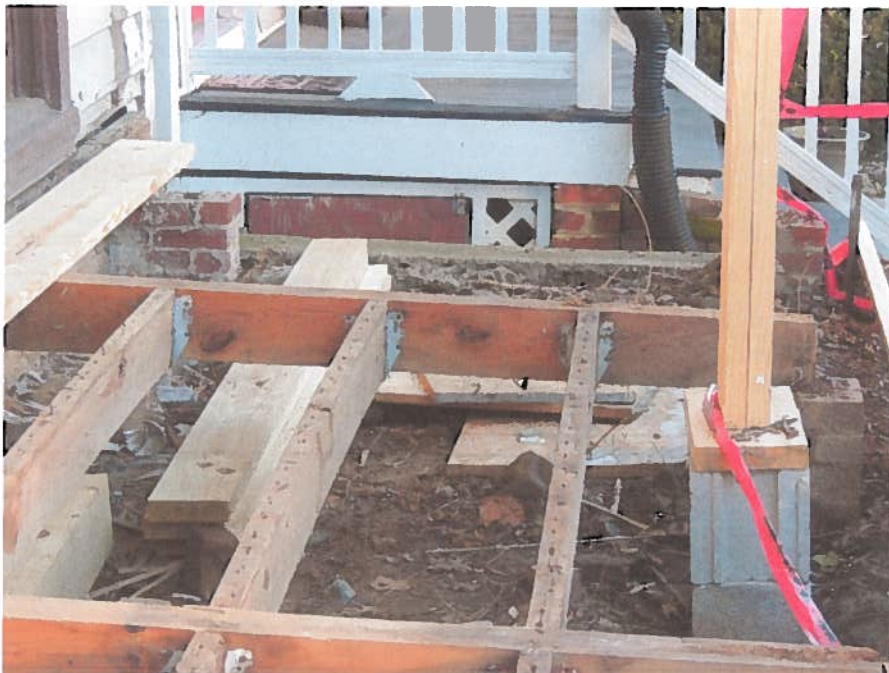
#11 floor joists not yet removed
