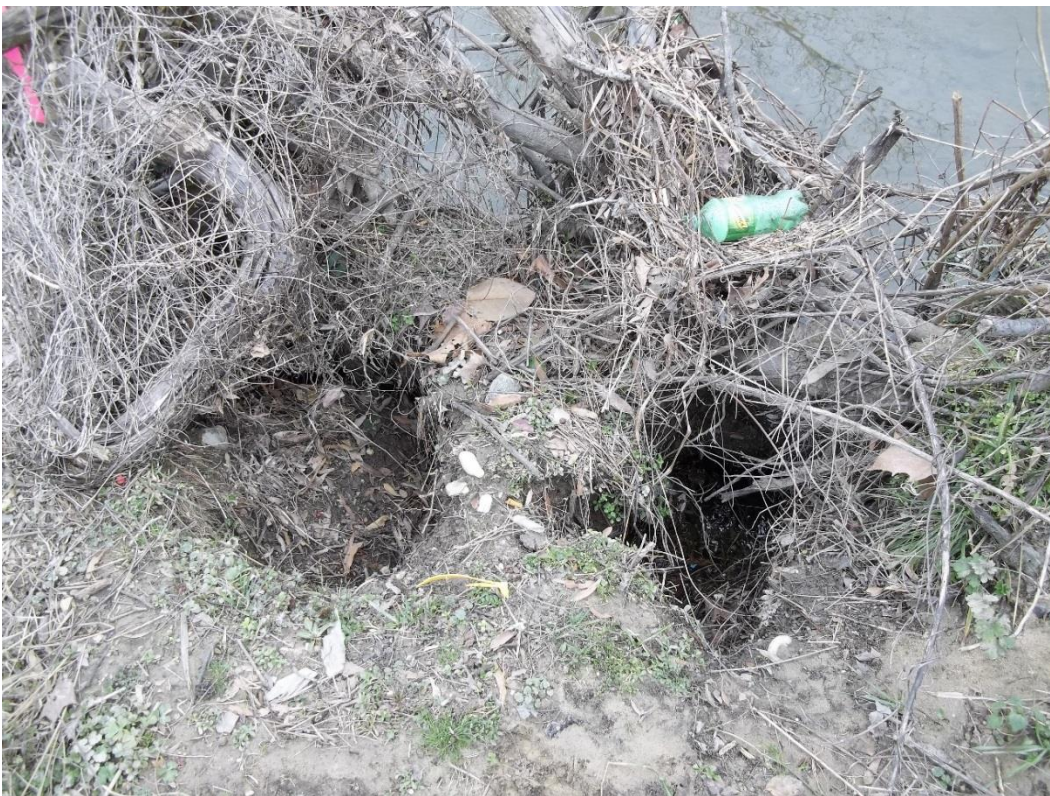
Erosion occurring behind buried root balls embedded in the left bank.
