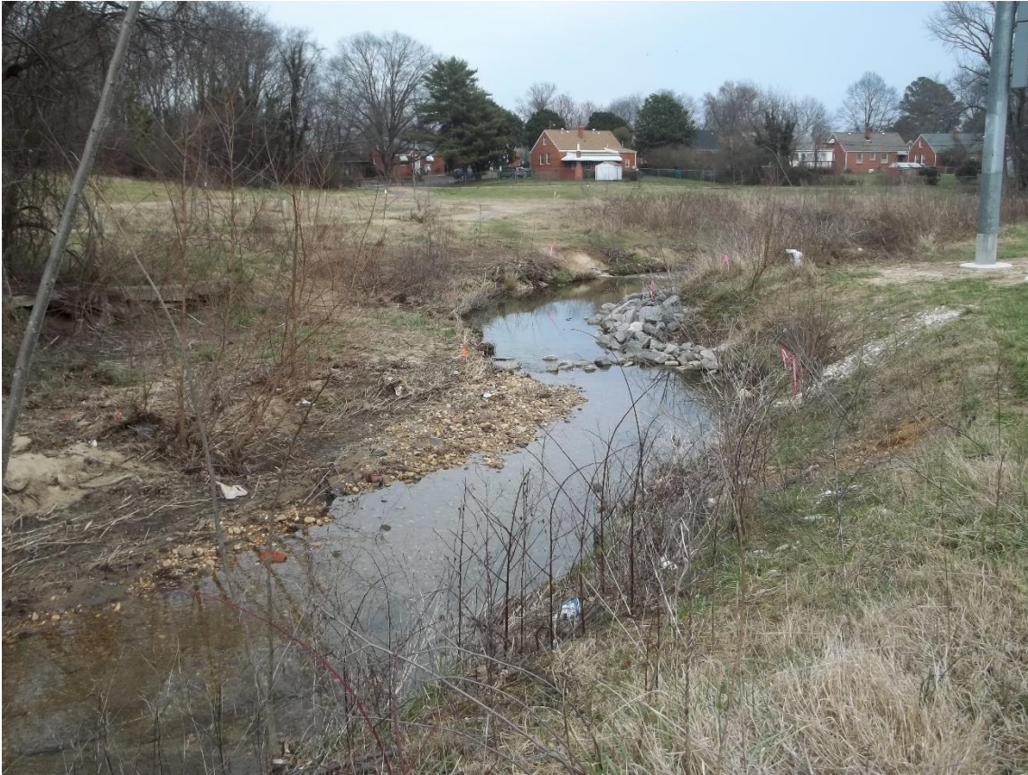
Overview of the upper end of the stream restoration. Note riprap piled along right bank at the first bend in the restored area. This stopgap measure was taken after this segment of the stream restoration failed shortly after installation.
