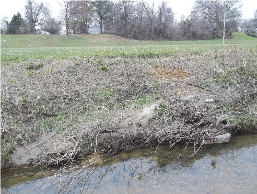
Erosion and damaged matting along right bank.
