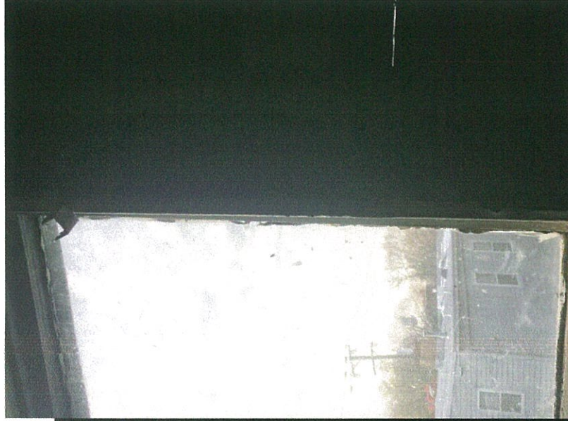
#3 window does not open and has rotted
