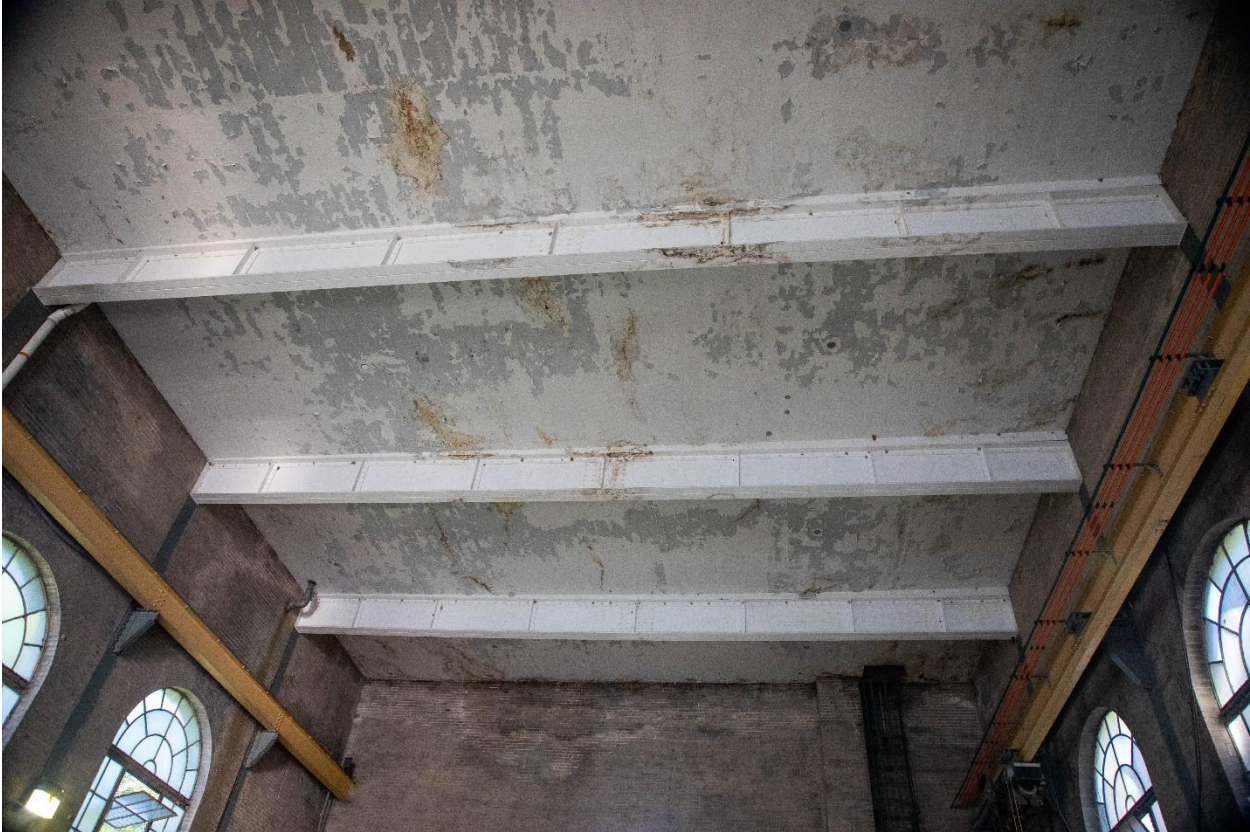
Water leaks through the roof structure.
