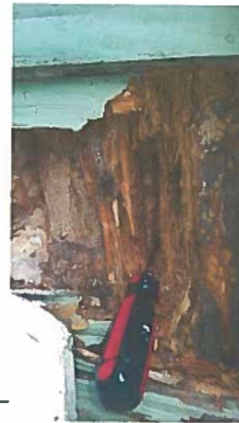
Deterioration of the front wall of the house is significant. Evaluation of the extent of damage is proposed during the demolition of the porch. Repair and reinforcement of the front wall framing is necessary for the structural integrity of the house
