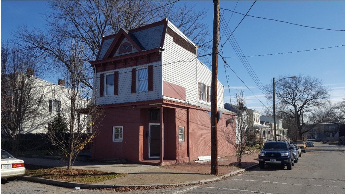
PHOTO 1 WEST / FRONT – SOUTH / SIDE ELEVATION VIEW FROM ROUNDABOUT AT CHIMBORAZO BLVD. & E. MARSHALL ST.
