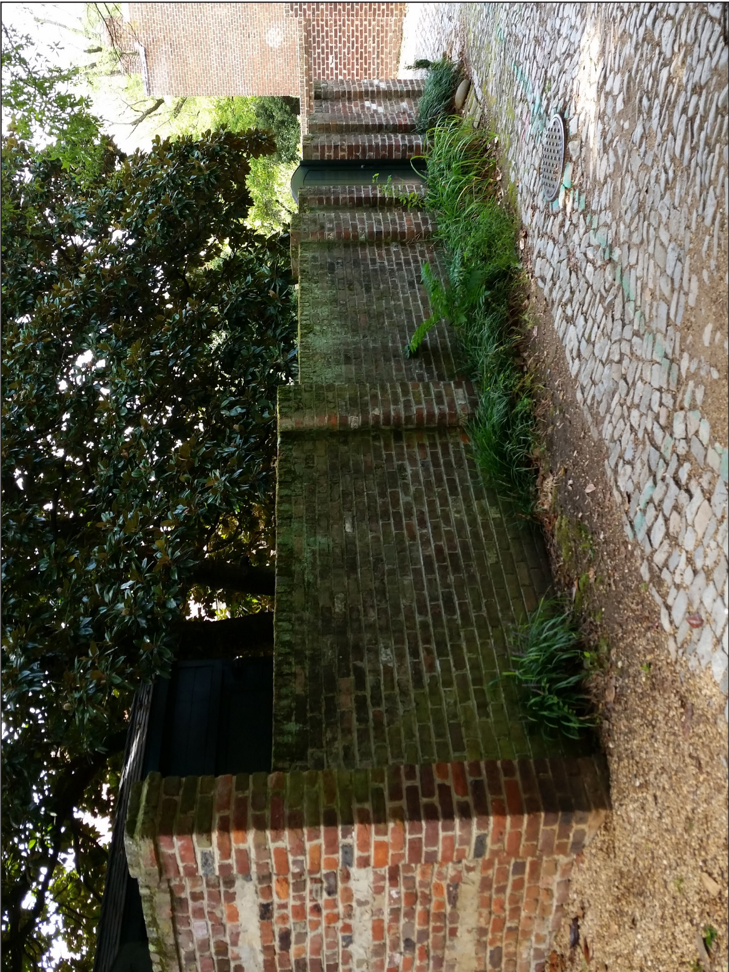
Example of proposed wall, located in the N. 23rd-24th Streets' alley, between E. Broad St and E. Grace St.
