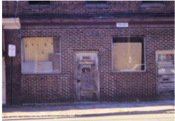
Figure 2. 411 Brook Road, 1997. Storefront infilled with brick. Poor condition. Original materials and configuration have been removed/altered.
