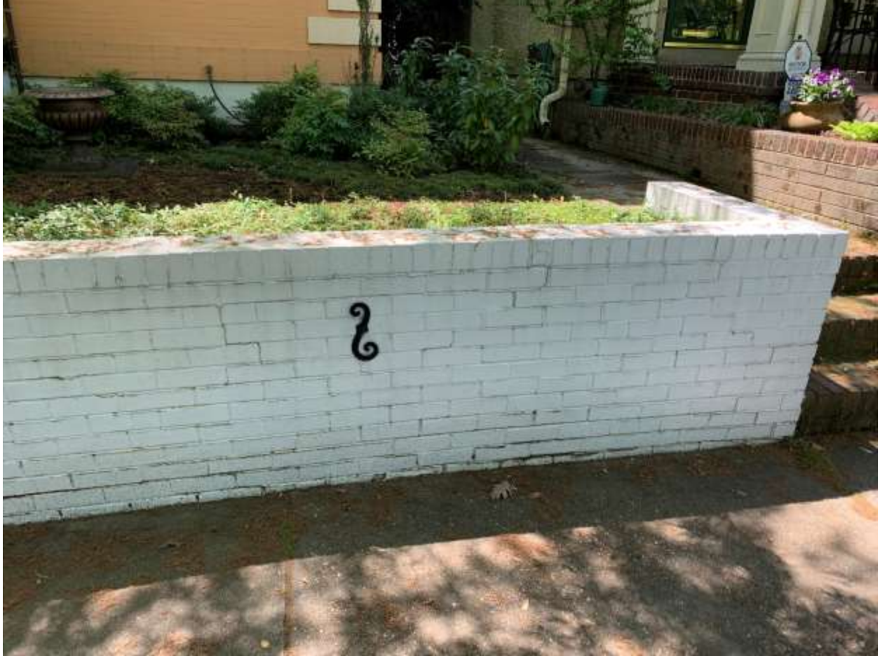
Structural Cracks at Front Retaining Wall- Right Side
