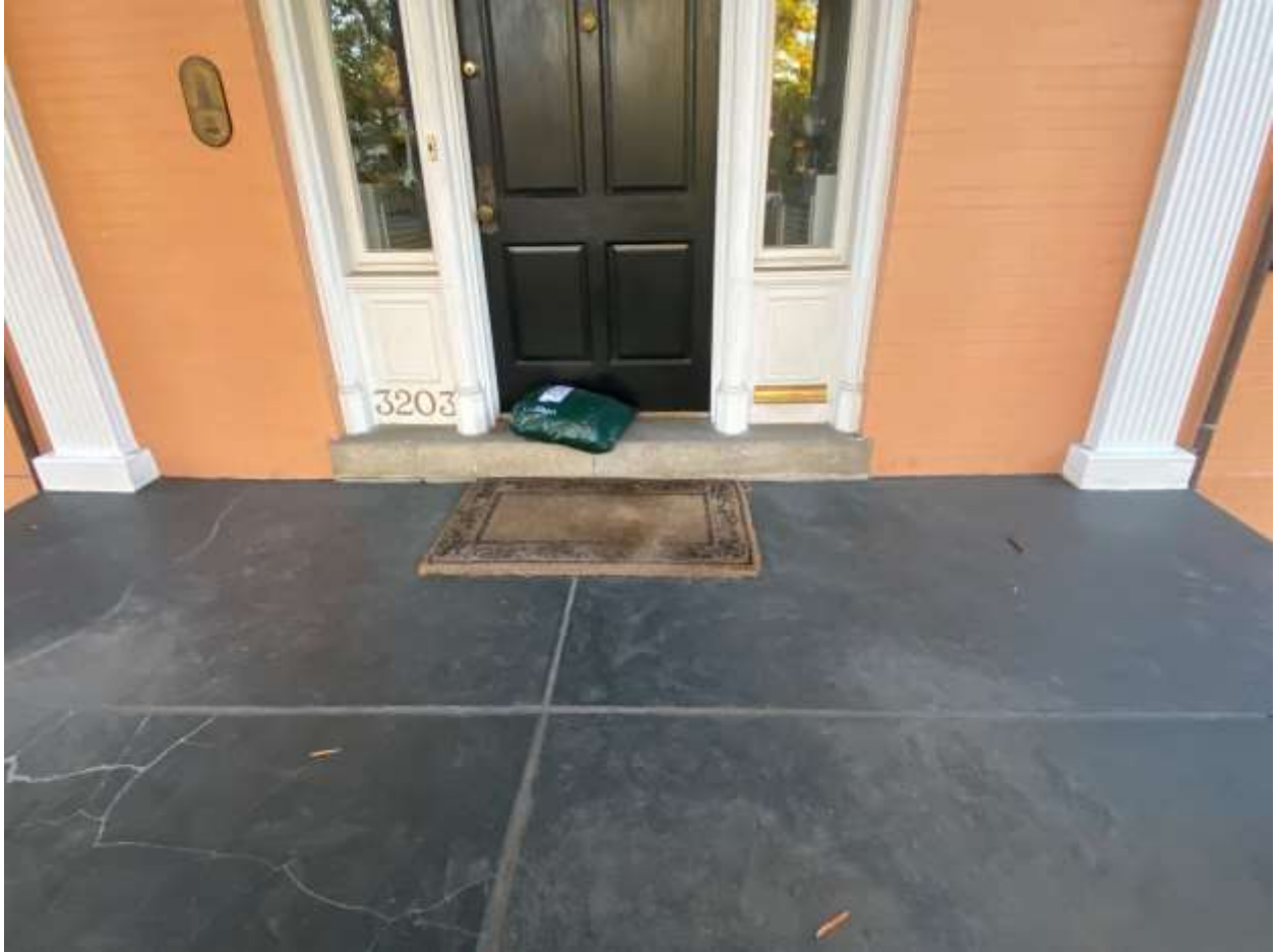
Top of Porch Showing Structural Cracks and Sunken "Bowl"
