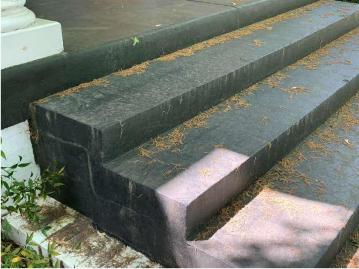
Concrete Steps Showing Previous Repair Attempts
