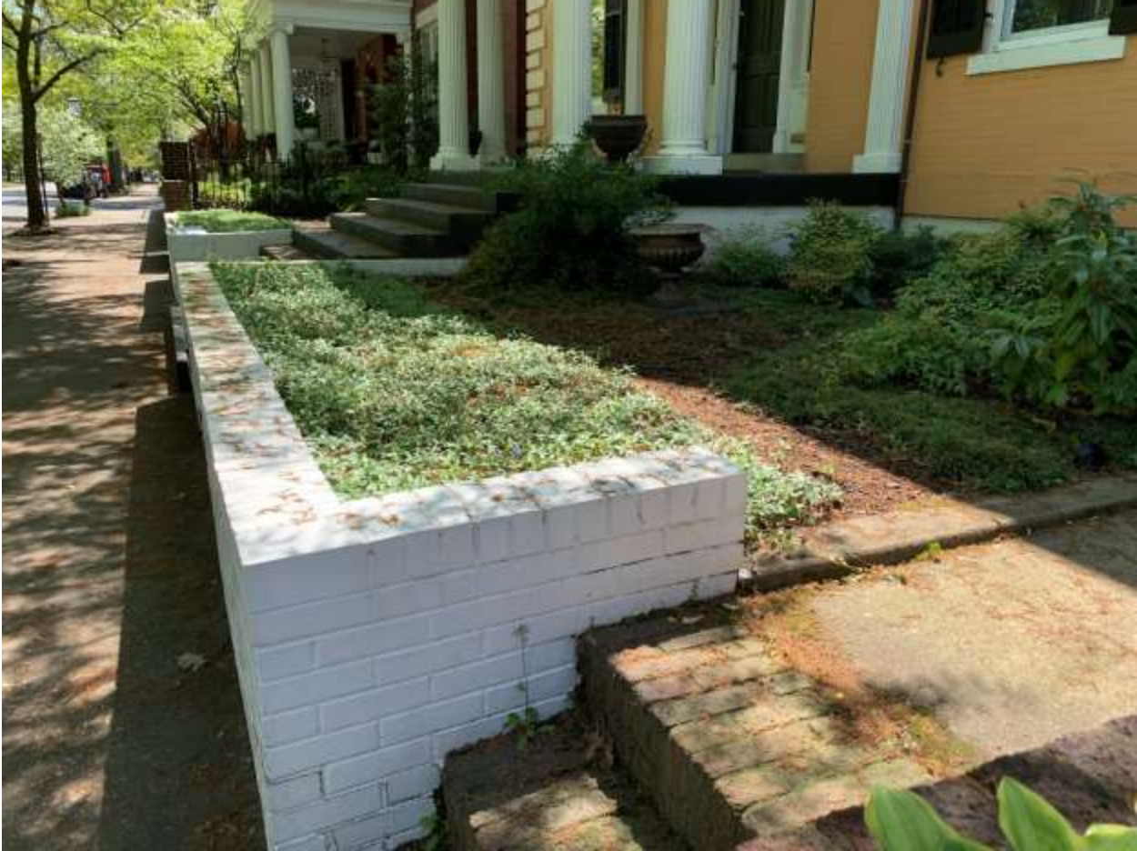
Retaining Wall Leaning into City Sidewalk
