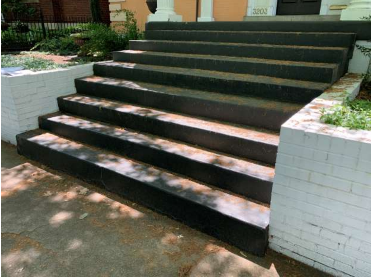
Concrete Steps Showing Inconsistent Treads/Risers and Structural Cracks
