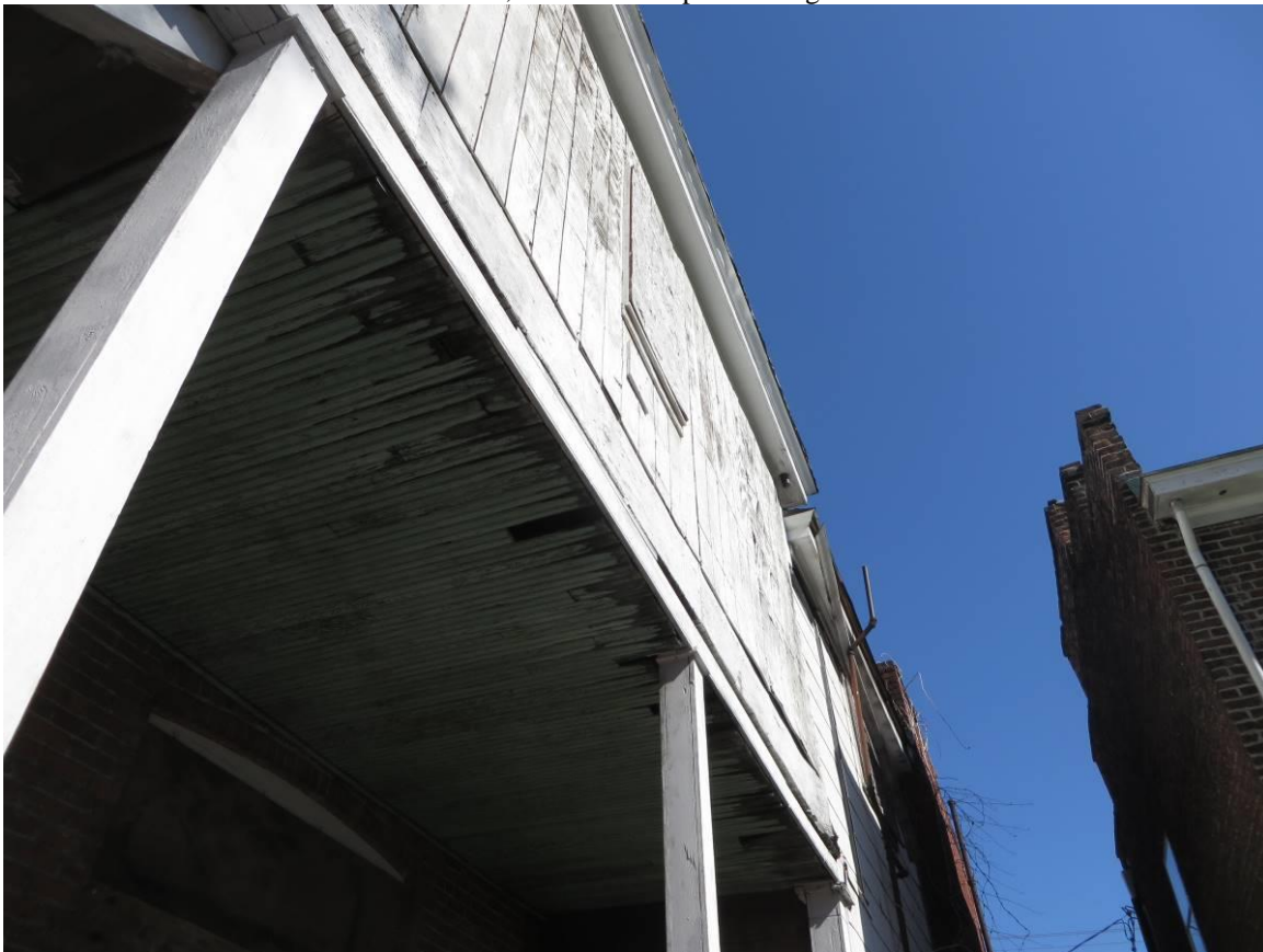
Photo 6: East elevation, view of the plywood siding at the enclosed second floor level
