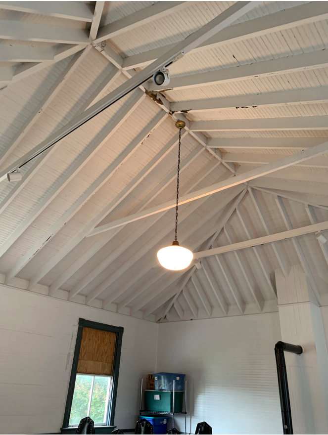
Interior image showing water damage
