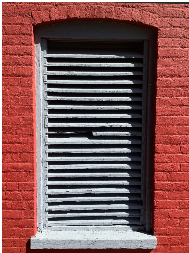
Example of damage to exterior louver
