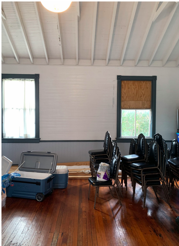
Interior detail showing window damage
