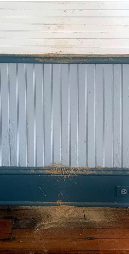
Detail of insect damage
