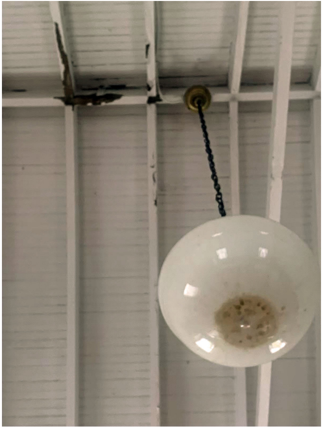
Interior image showing water damage
