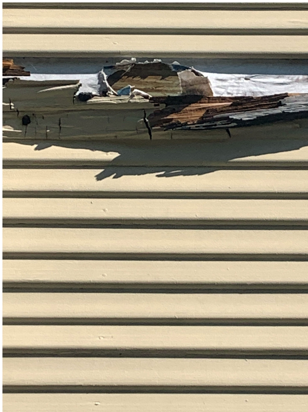
Example of damage to exterior siding
