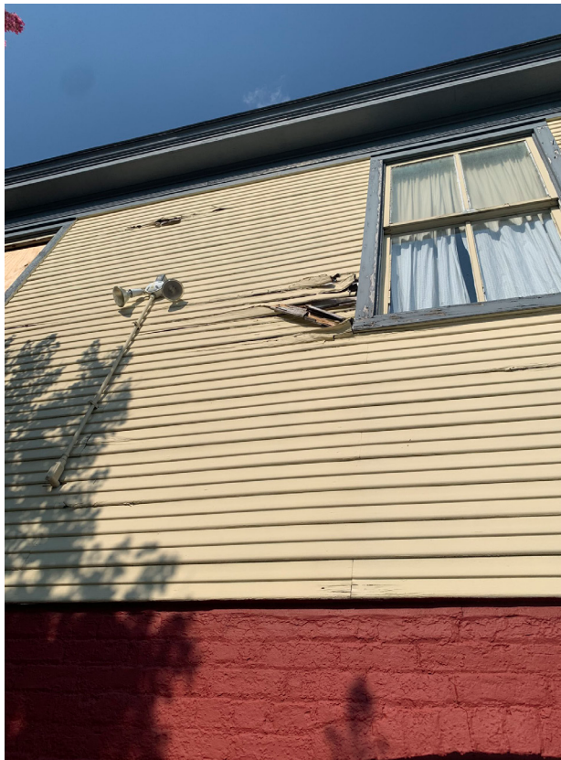
Damage to exterior siding
