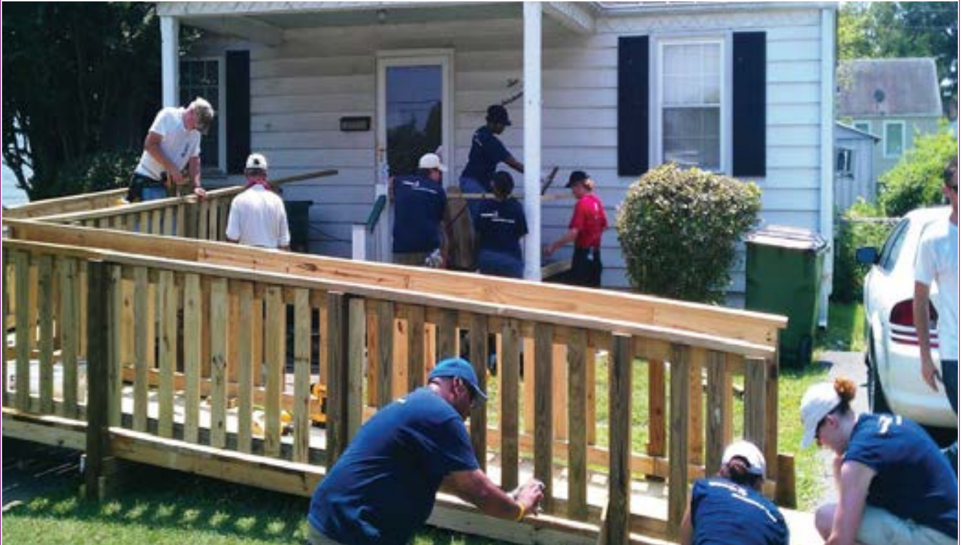
Project: HOMES - adding a ramp to allow residents to age in place.
