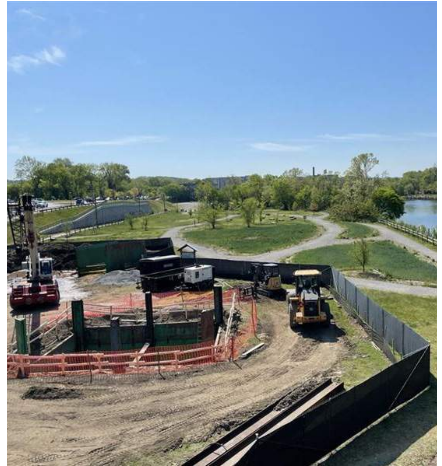
Southeast View from JRA, Dept. of Public Utilities Infrastructure Construction Spring 2026-Fall 2026
