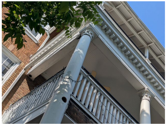
Figure 6. Existing condition of eastern column. April 2026.
