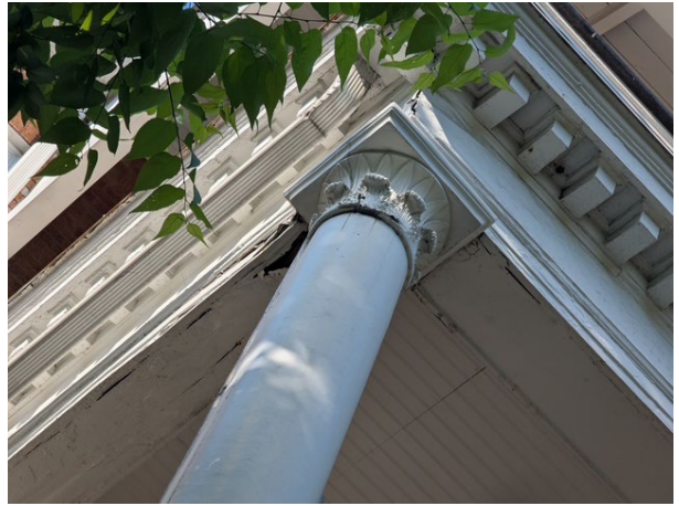
Figure 4. Existing condition of eastern column. April 2026.
