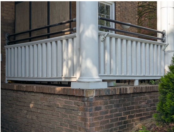
Figure 7. Existing condition of eastern column. April 2026.
