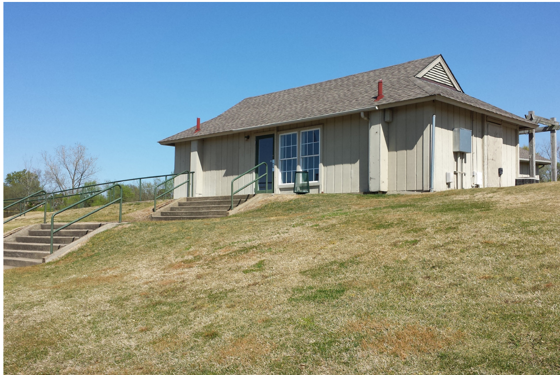
Small building and site stairs to be demolished to accommodate new accessible ramp, stairs, and pedestrian entry
