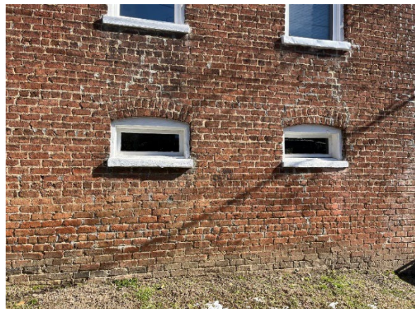
Figure 4. Existing transoms at basement level on the alley elevation. These appear to be original to the building.
