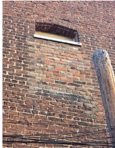
Figure 2. Window that has been infilled without approval. Sill relocated and infill toothed into original masonry.
