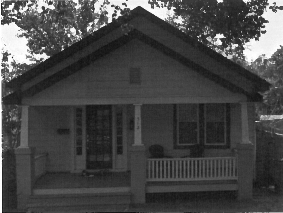
This is the state of the home in 2010. The sidelights were uncovered and the temporary door is in place. Notice the bowing piers and columns.
