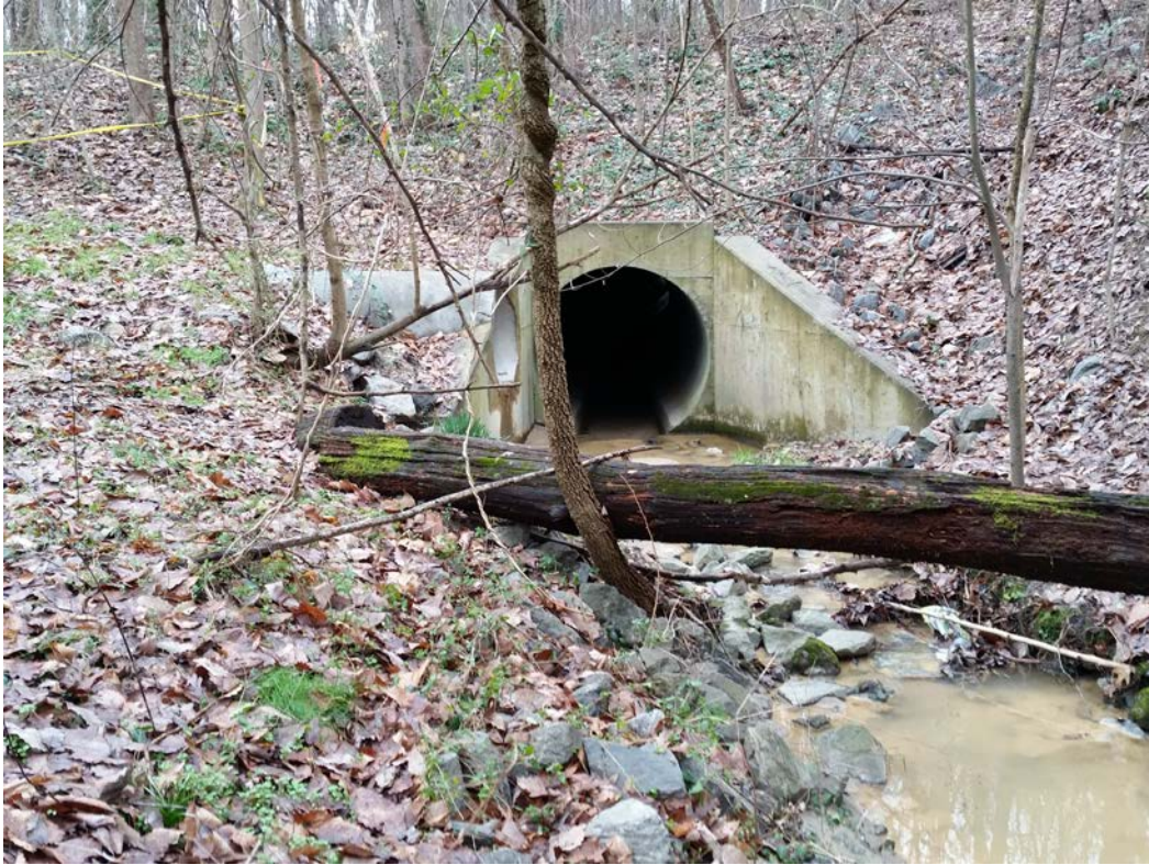
Downstream reach of perennial stream through 72" RCP on-site and storm pipe outfall from adjacent Riverside Heights subdivision
