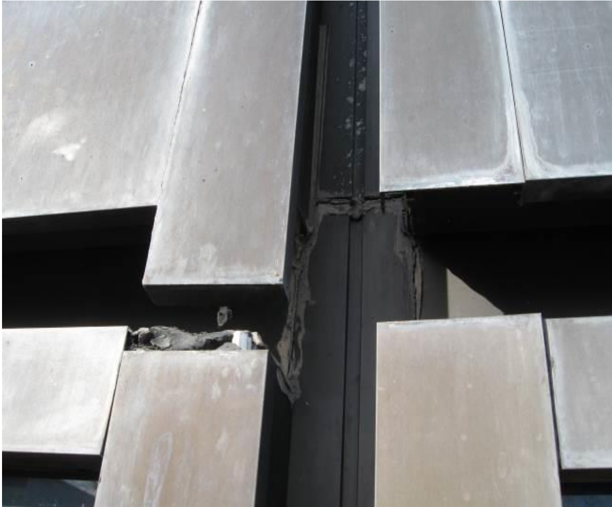
Figure 15: The vertical face caps are dropping downward and it can be seen where repeated attempts at caulking may also be directing water into the interior space.
