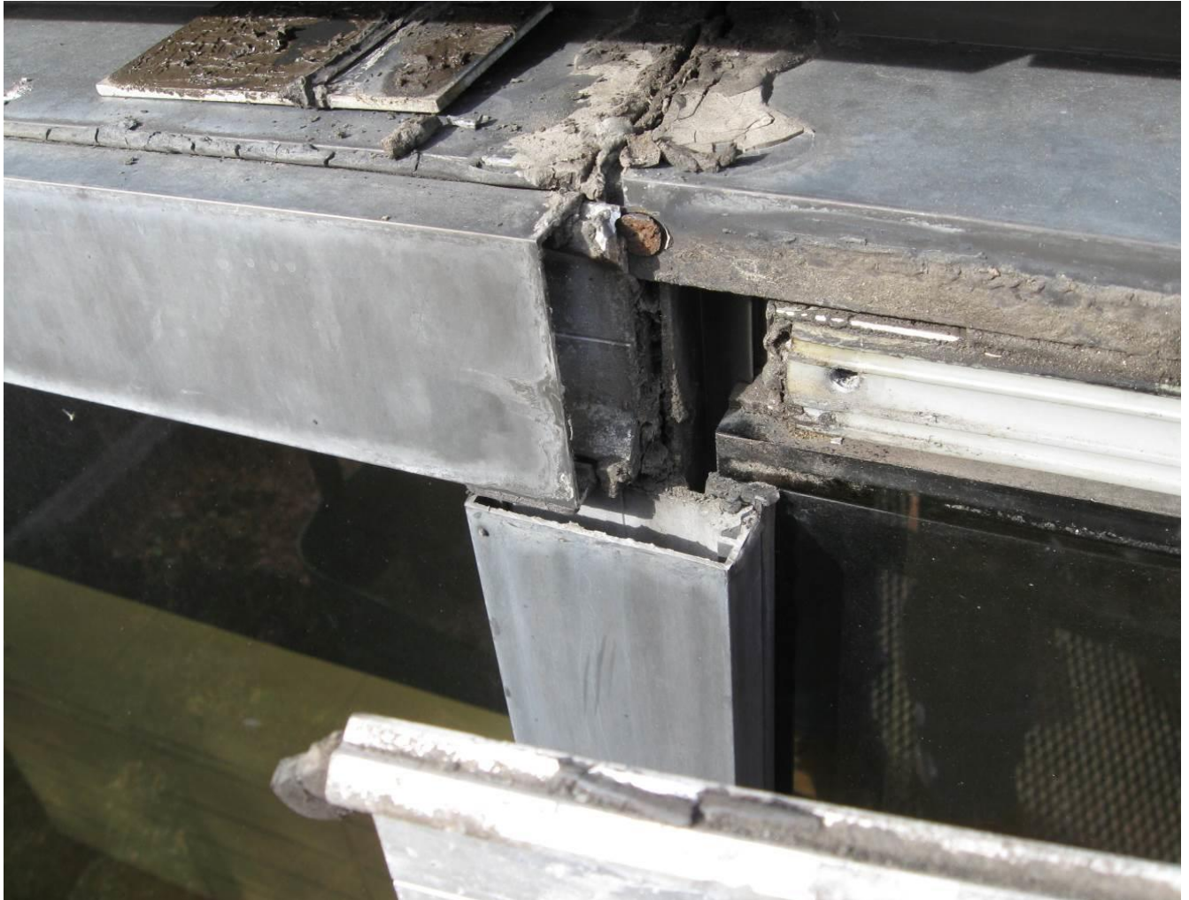
Figure 3: This close-up view of the exterior horizontal and vertical frames with one of the face caps removed provides a good view of the sealant. Note its condition: All the rubber and butyl tapes/seals and caulk/sealants are quite deteriorated.
