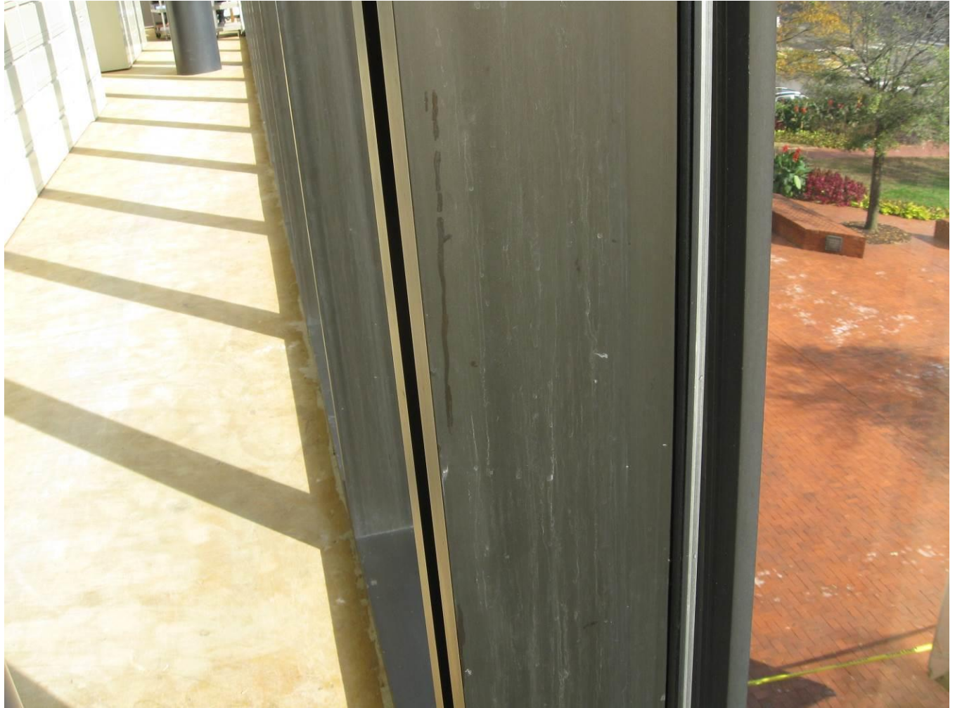
Figure 6: This interior picture shows that the existing window frames have water streaks and water stains.
