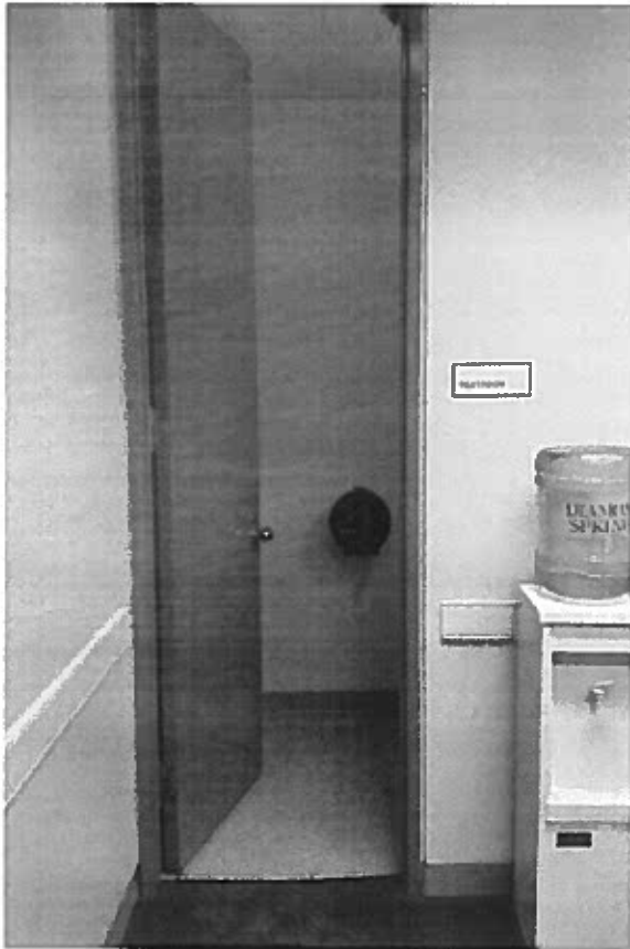
Door knob, signage incorrect, door clearance
