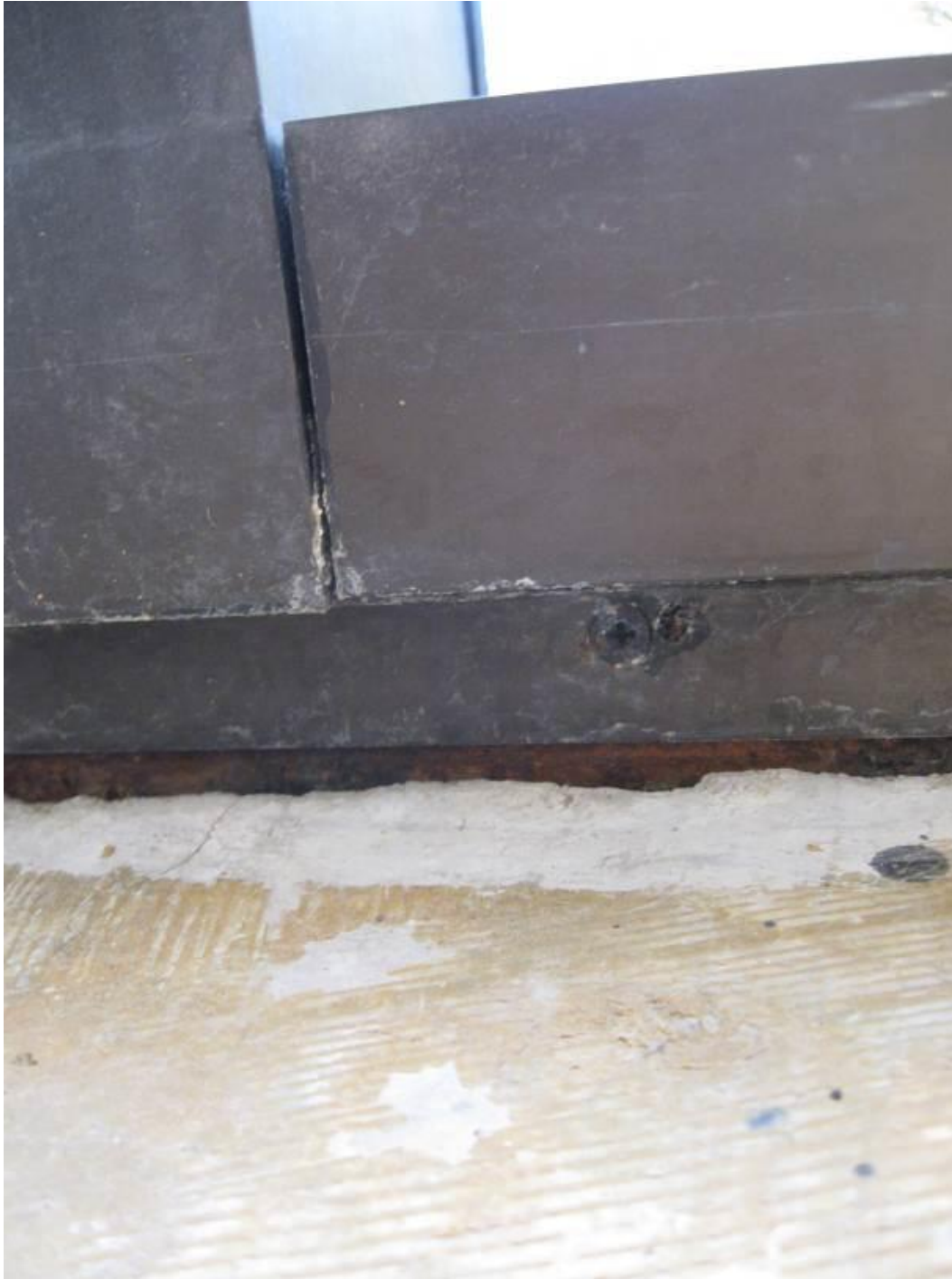
Figure 8 – This image shows the window sill at the floor slab as well as evidence of the structural member's rusting
