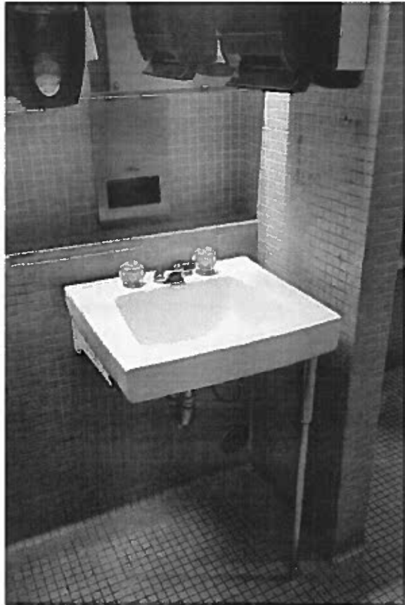
Clearance for sink approach, paper towel dispenser location and height, access to soap dispenser, uninsulated piping, faucet handles and sink support obstruction
