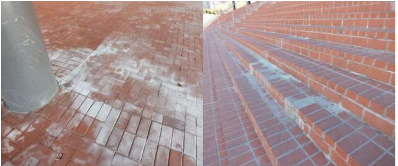
EFFLORESCENCE ON PAVERS
