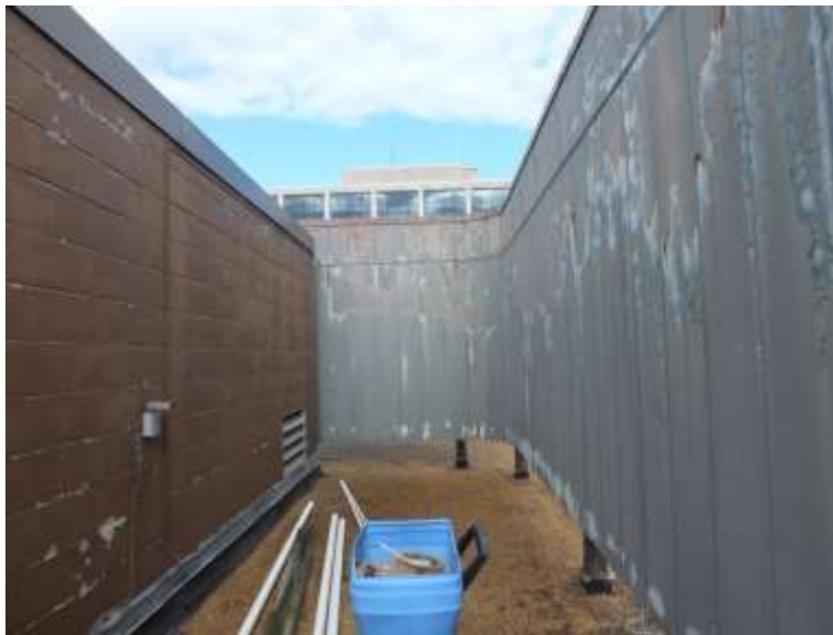
PEELING PAINT ON EQUIPMENT SCREEN AND PENTHOUSE
