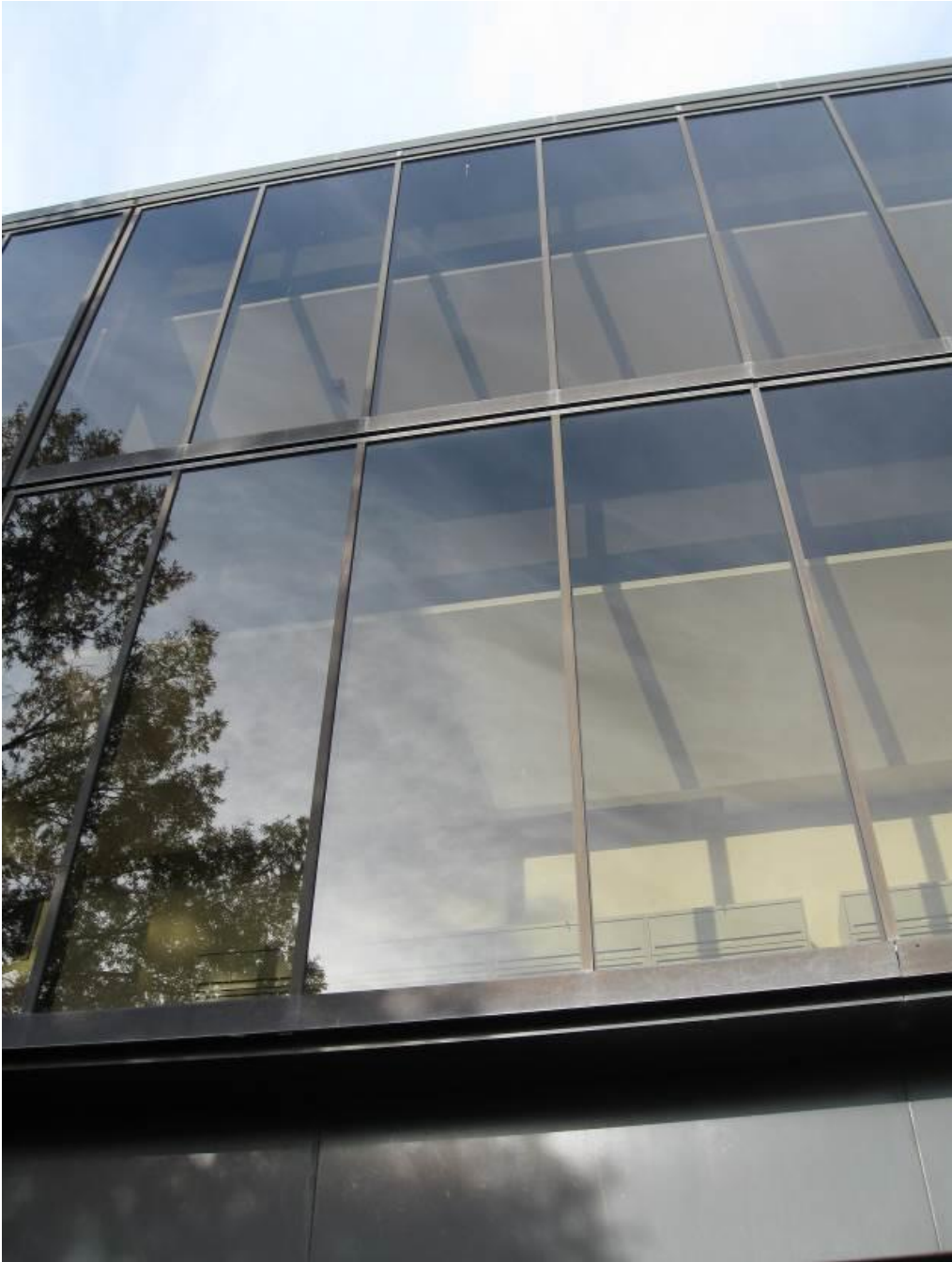
Figure 1: The existing curtain wall window system is an outside glazed system with a prefinished metal face cap.
