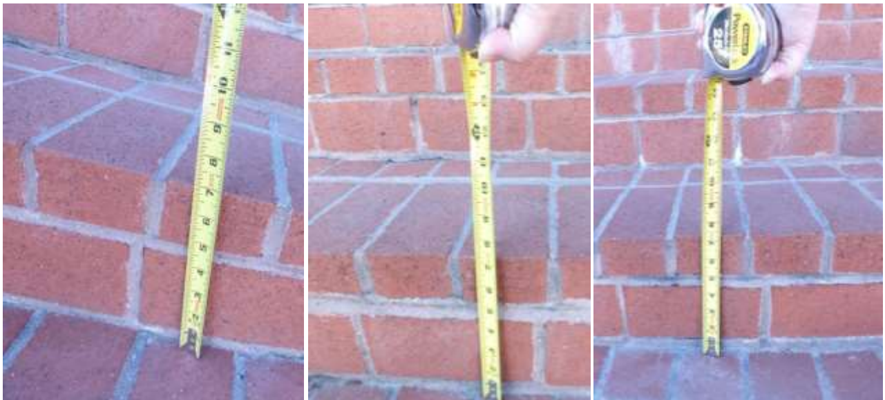
EXTERIOR STEPS - RISER HEIGHTS VARY
