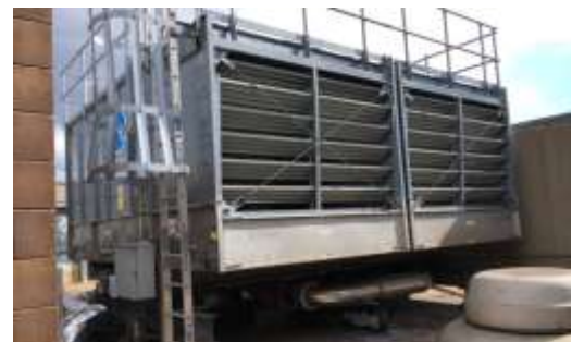
COOLING TOWERS, INSTALLED 2008
