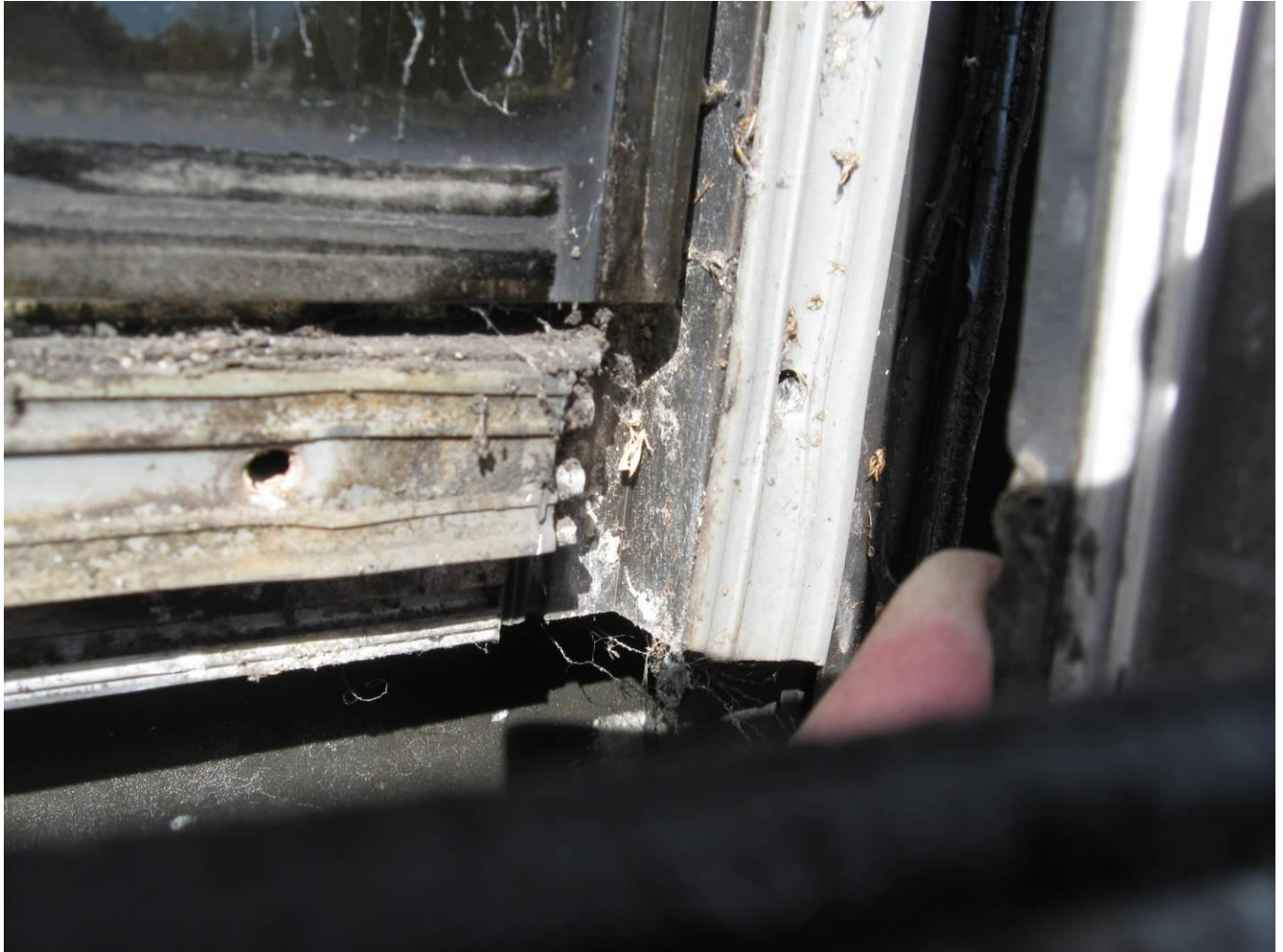
Figure 4: This is another view of a window at the expansion joint with the exterior face caps removed. Note that all the rubber and butyl tapes/seals and caulk/sealants were quite deteriorated.
