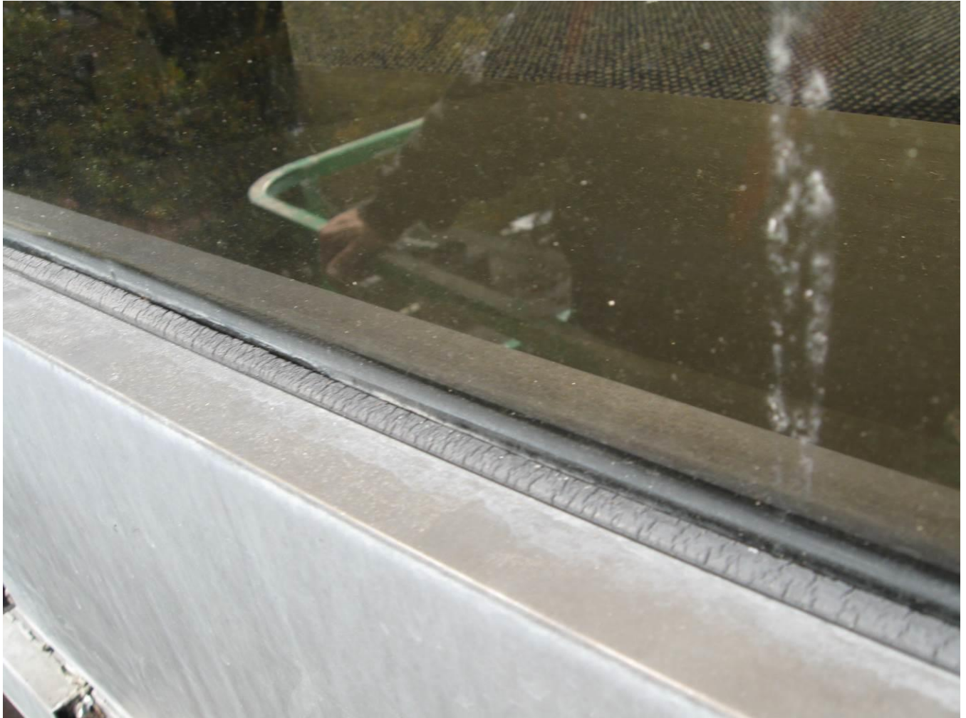
Figure 5: As this typical exterior picture reveals, the existing window gasketing/seals show deterioration, cracking, and exposure.
