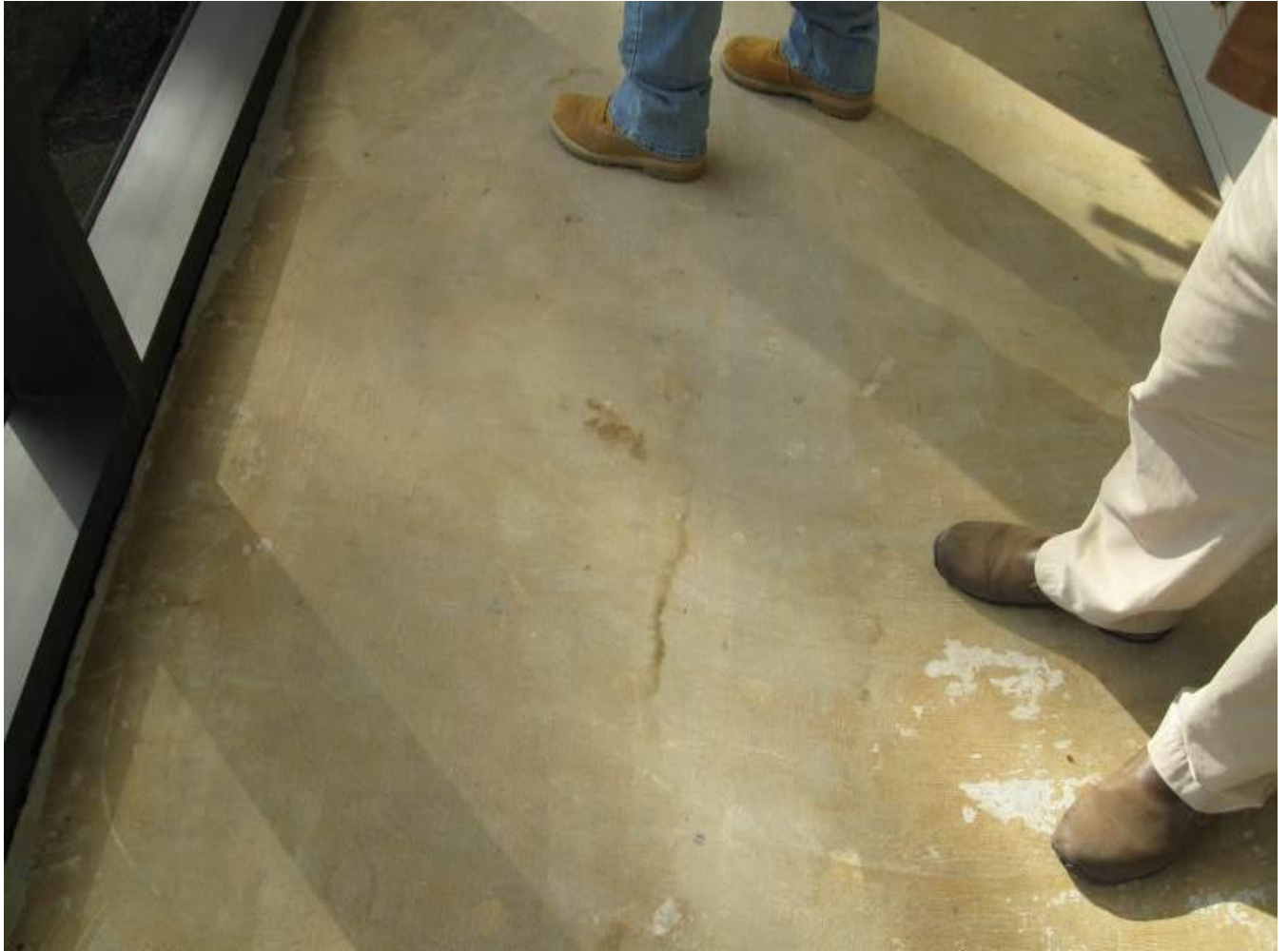
Figure 7: This interior picture shows water stains and water spots on the floor.
