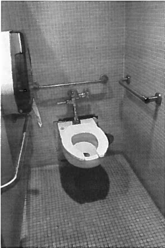
Stall too narrow, lack of clearance, mounting height for toilet paper dispenser, incorrect grab bars
