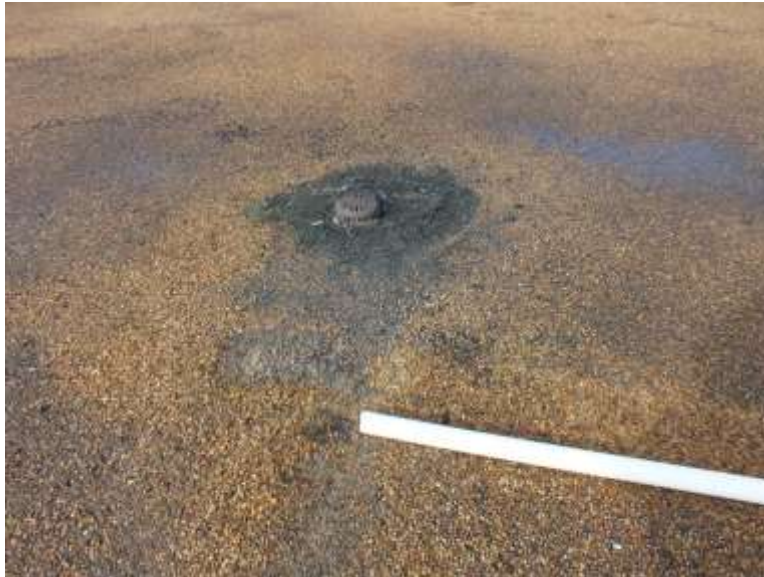
PONDING ON ROOF
