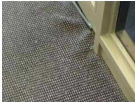
BROADLOOM CARPETING BUCKLING
