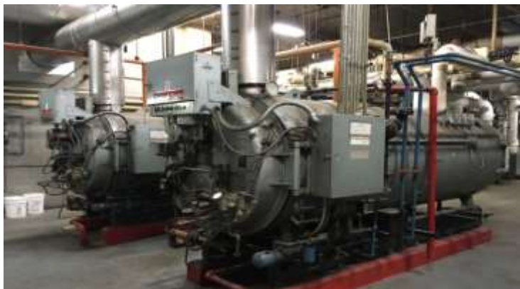
BOILERS, INSTALLED IN 1975
