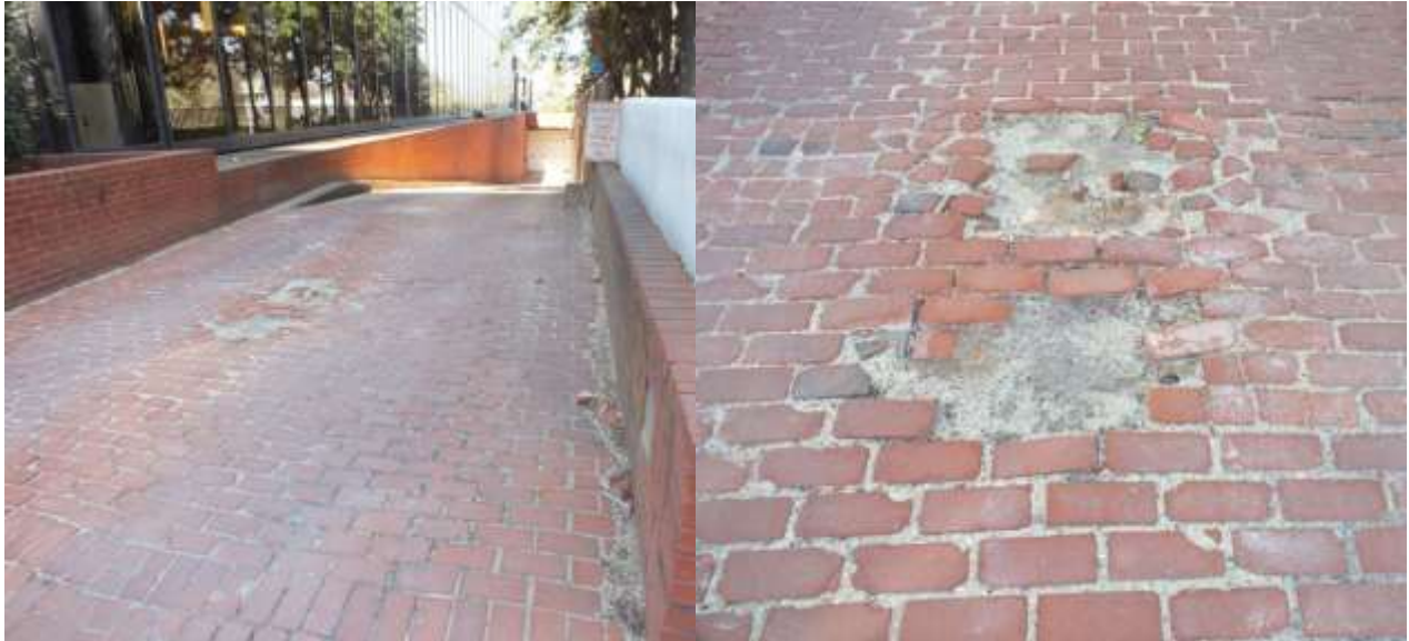
LOADING DOCK RAMP - UNEVEN AND MISSING PAVERS
