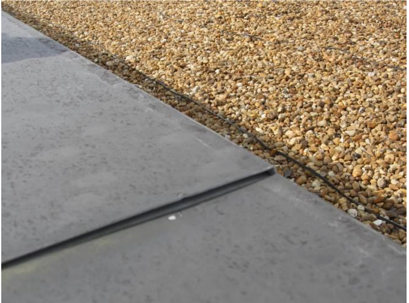
Figure 10: The top of the coping is not as tight as it should be.
