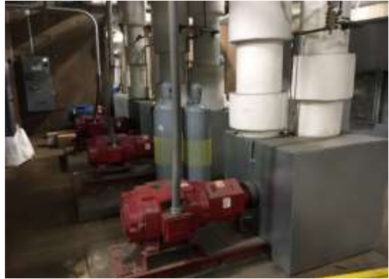
CHILLED WATER & CONDENSER WATER PUMPS
