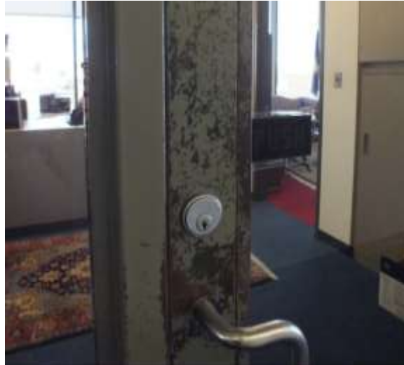
DAMAGED FINISH ON DOORS
