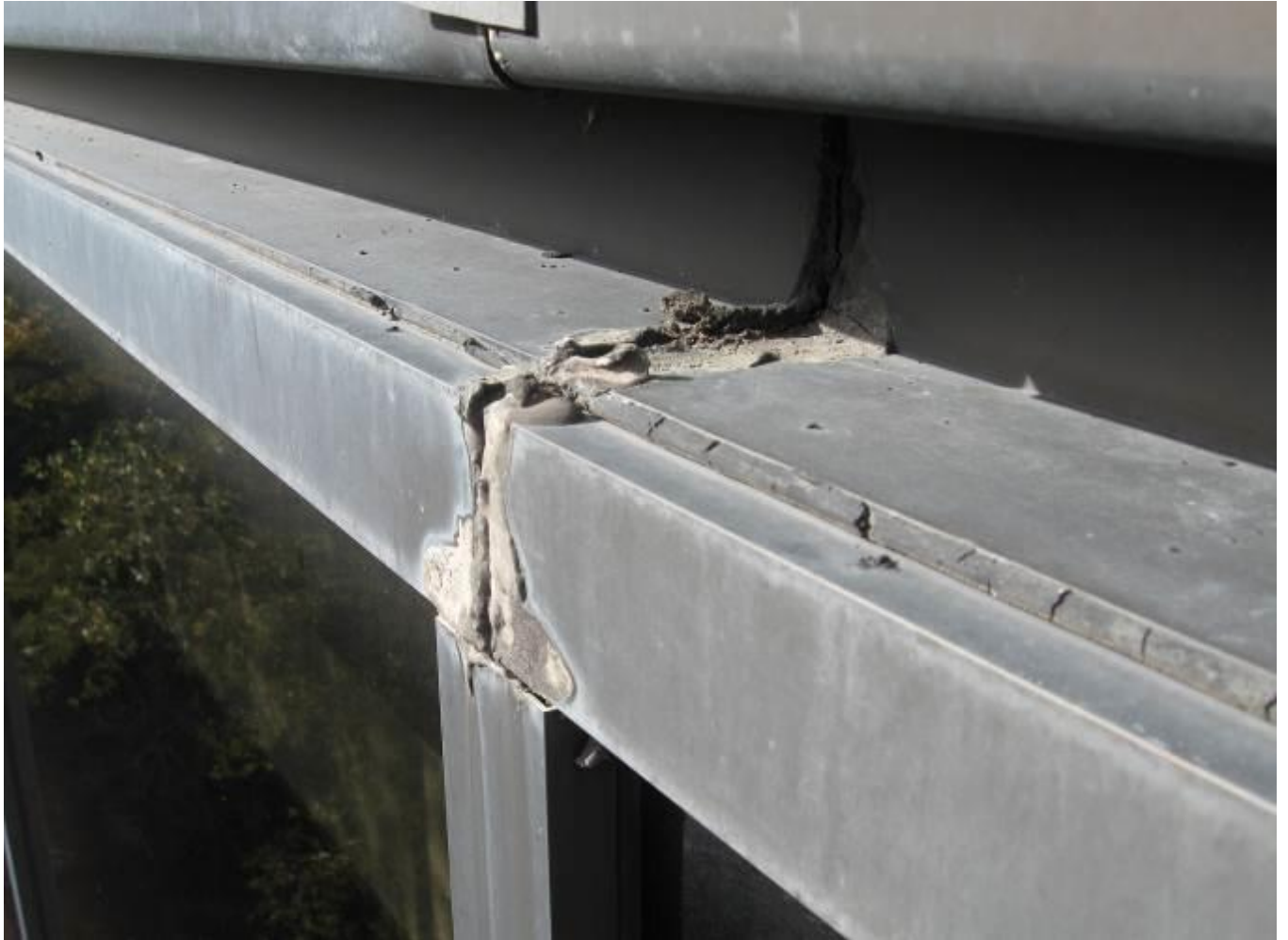
Figure 12: As shown in this photo, repeated attempts were made to caulk and patch the top-most window frame.
