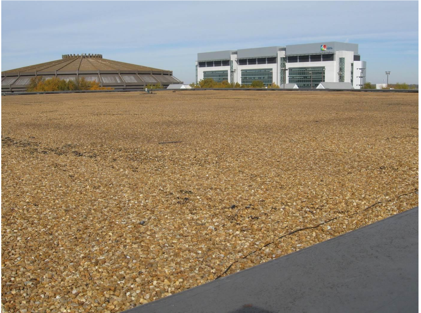
Figure 13: The 40-year-old roof appears to be in fairly good condition despite its age.
