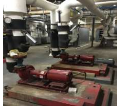
HEATING HOT WATER PUMPS
