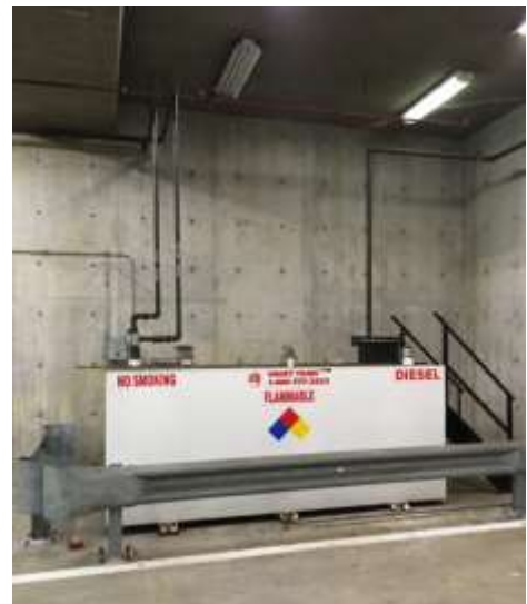
FUEL OIL STORAGE TANK
