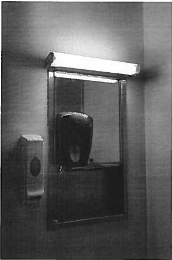
Mirror obstruction & dispenser height
