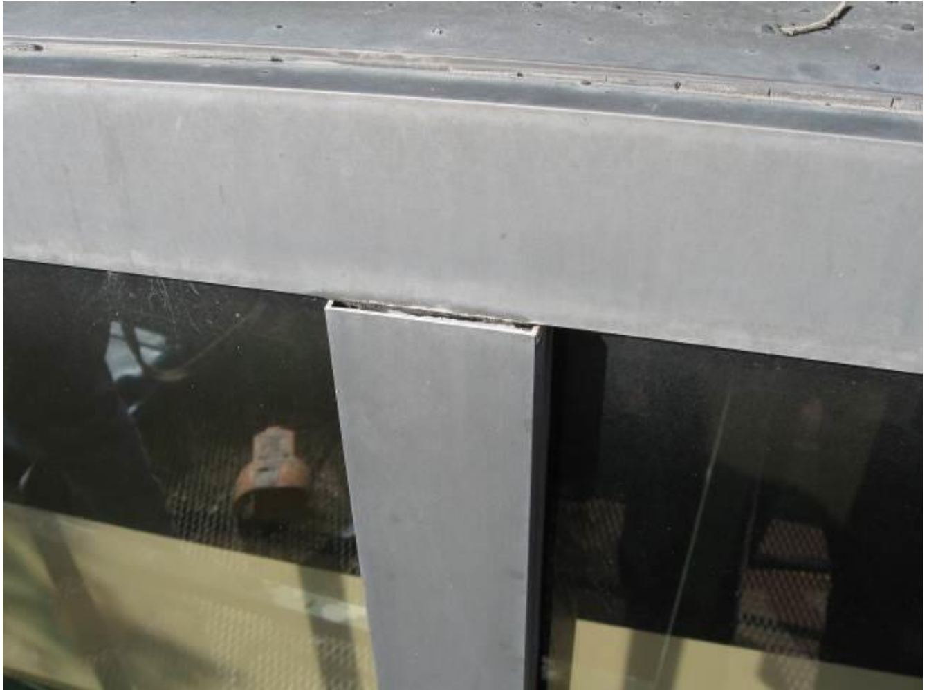
Figure 14: The face cap is pulled away from the window. The resulting gap exposes the interior to the elements, if the seals and flashing have failed underneath.
