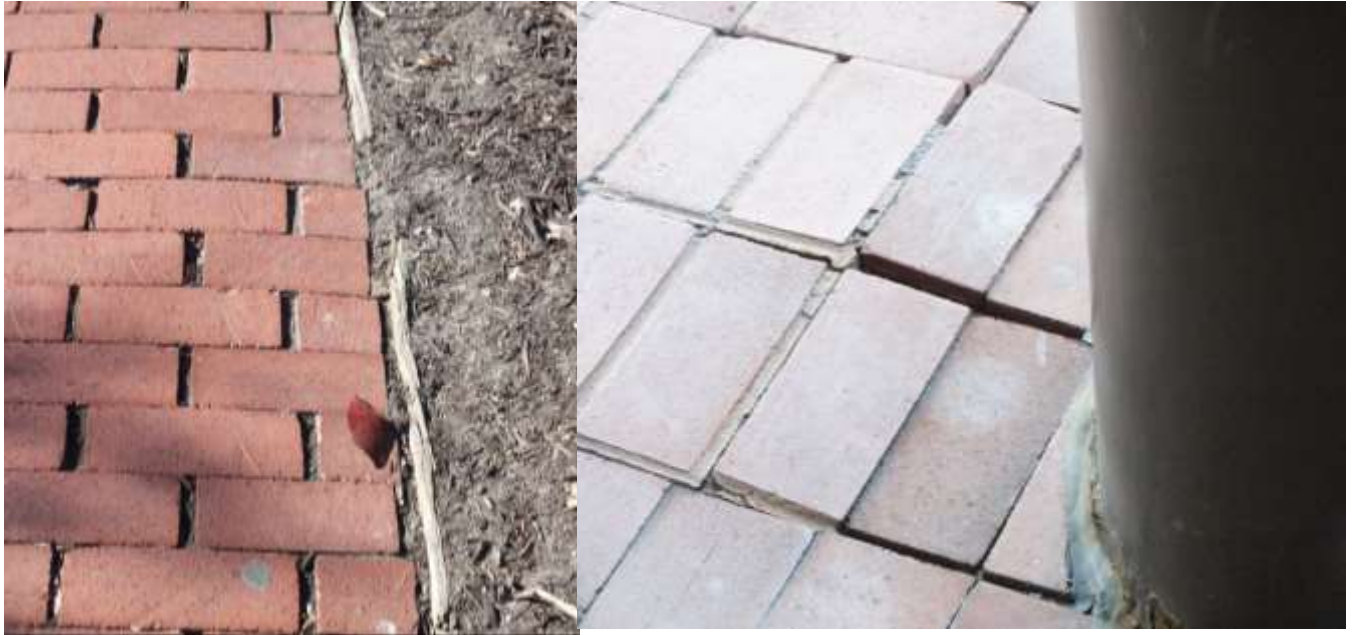
BRICK JOINT SEPARATION
