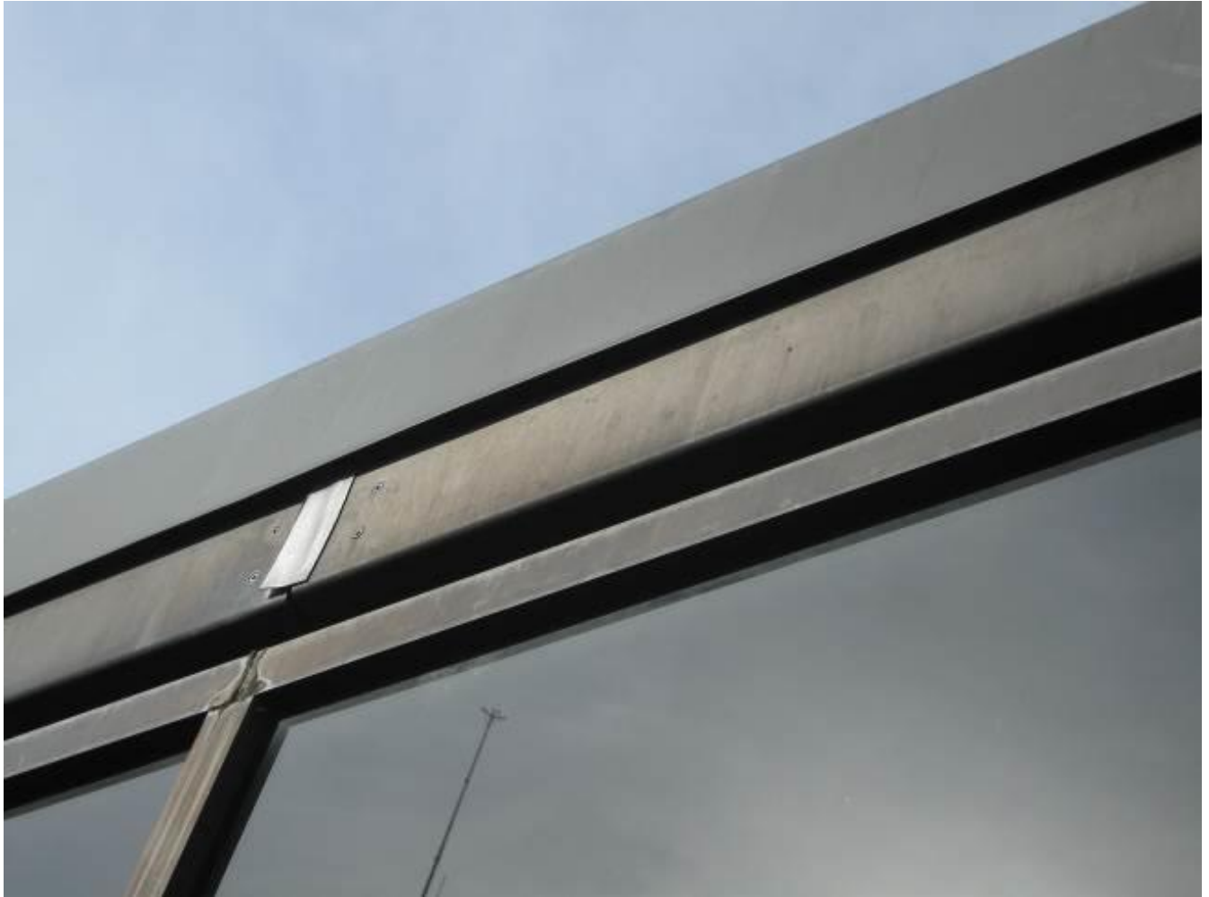
Figure 9: The metal coping shown is typical for the perimeter of the building. The upper most band is the metal coping (vertical leg). The band below that coping is most likely a prefinished metal panel covering the structure, which may be part of the window system. Below that is a gap and then the window frame.
