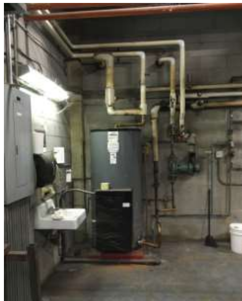
ELECTRIC DOMESTIC WATER HEATER
