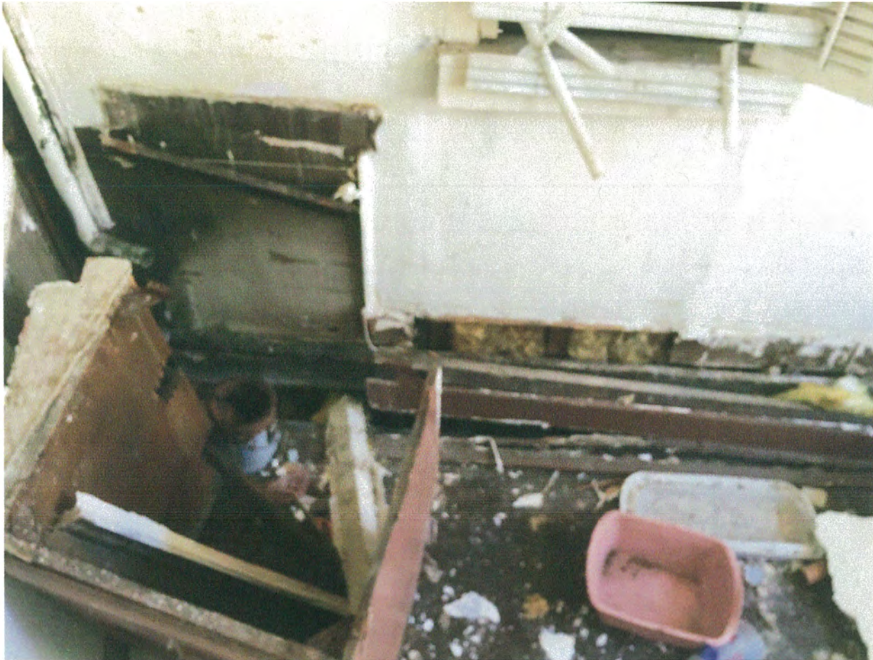
Bathroom floor sloped and needs to be completely rebuilt
