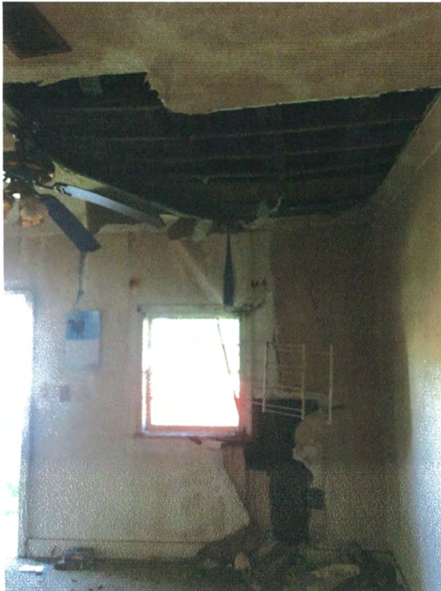
Plaster detached from ceiling due to water damage.
