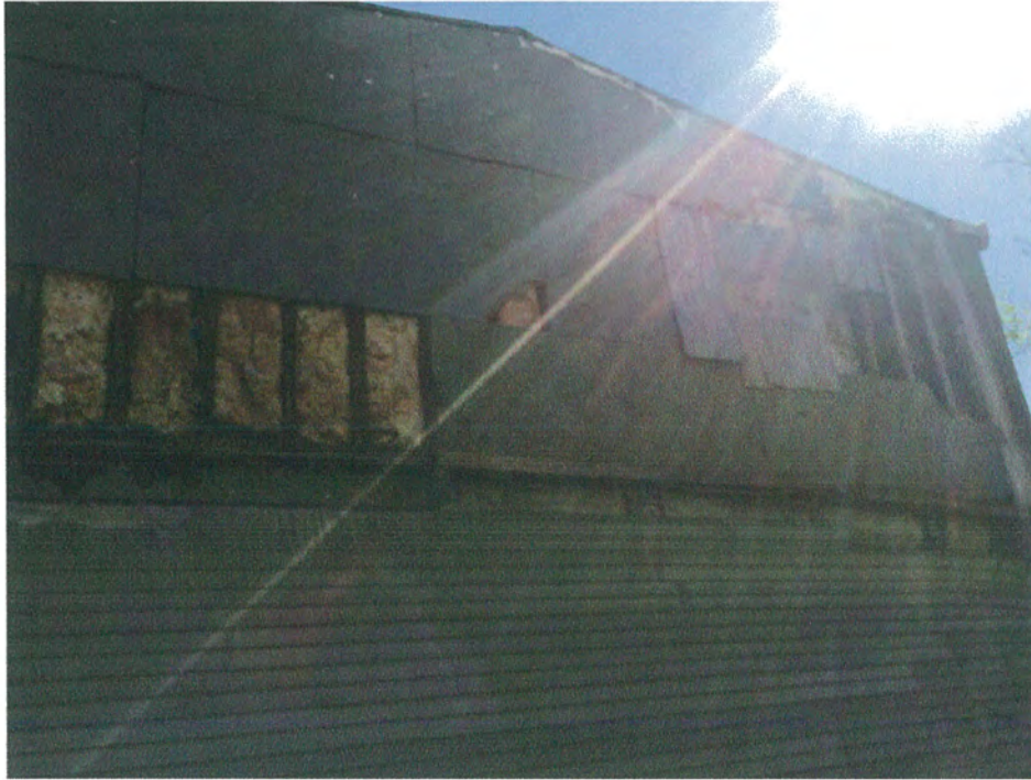
Exterior wall completely exposed to the outdoors
