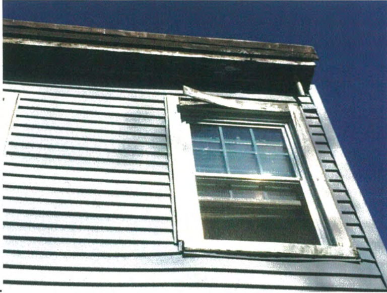
Complete replacement of soffit, fascia and window trim. Current windows have grids but are not simulated divided lights.
