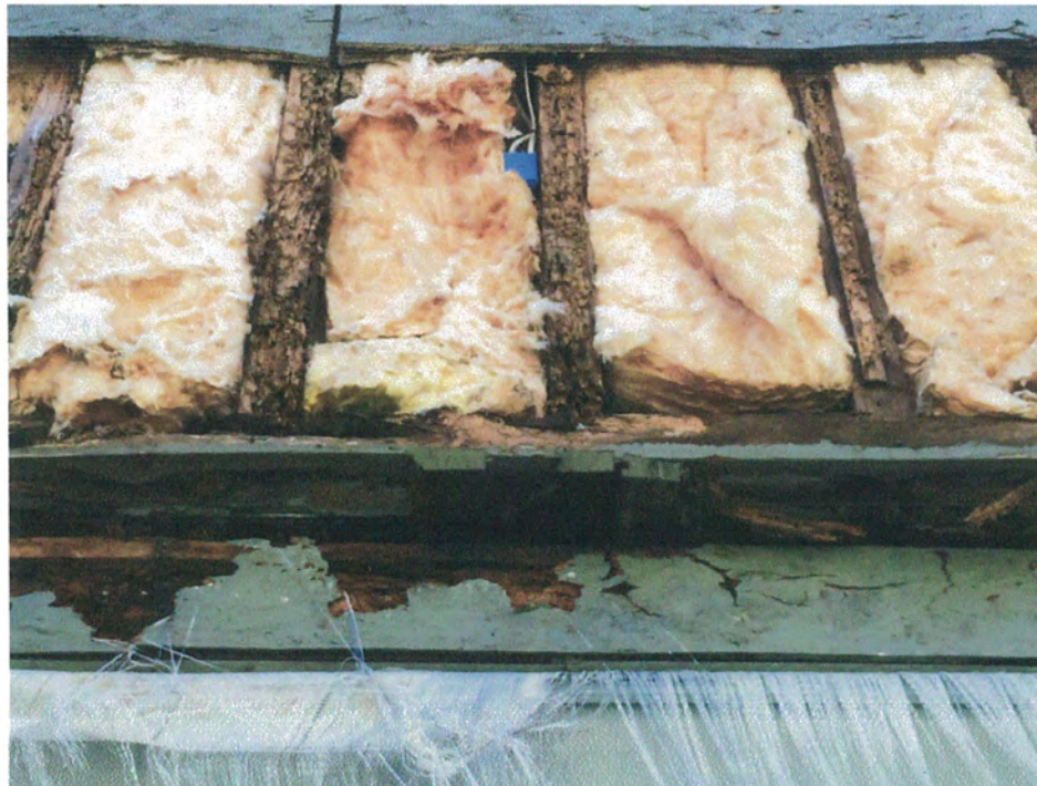
Floor Joists and studs completely rotted
