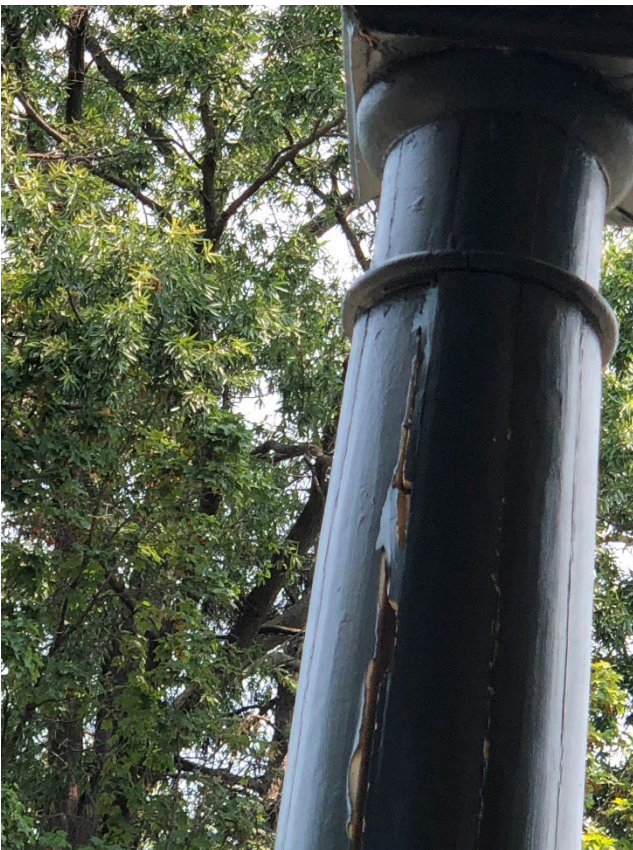
Figure 7. View of deterioration on the far west column.
