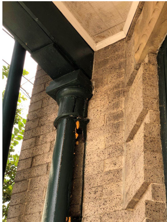
Figure 8. View of deterioration of the top of the east engaged column.
