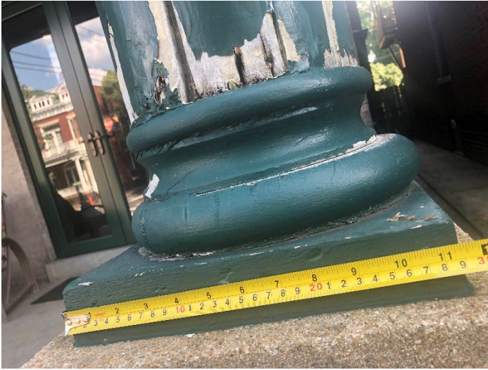
Figure 5. Close-up photograph of deterioration on the base of the far west column.
