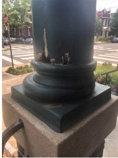
Figure 6. View of deterioration on the second column from the west.
