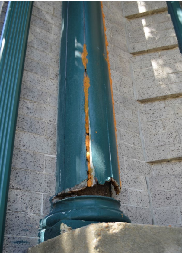
Figure 9. Photograph showing the deterioration of the east engaged column.
