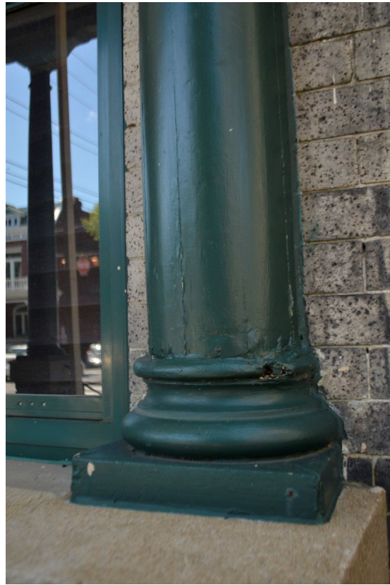
Figure 10. Photograph showing deterioration on the west engaged column.
