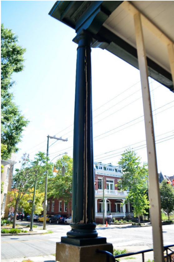
Figure 3. Photograph showing deterioration on the far west column.
