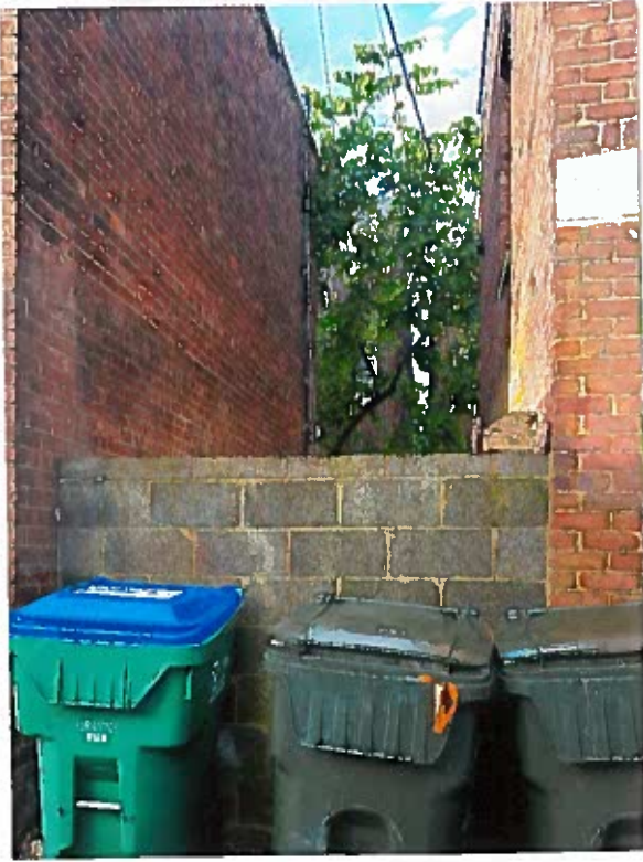
From alley - @ side of garage - plan to raise wall to 6'6" + place door for new alley entrance
