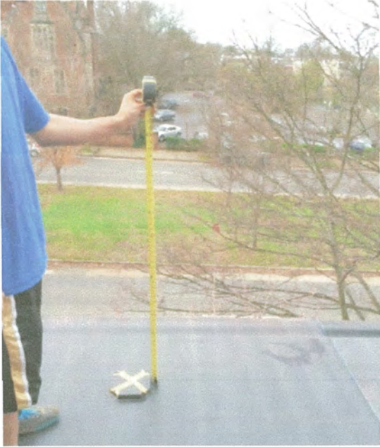
Newel post sit back over 2' from all edges. This is the exact original locations of newels.
