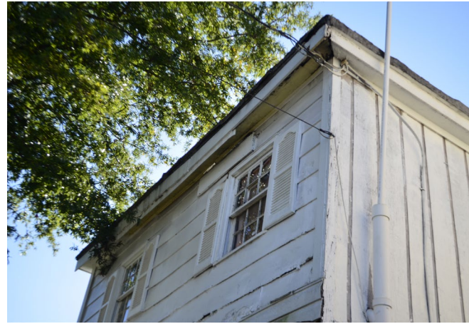
Figure 6. View of the poor condition of the foundation on the west side of 2417 Carrington Street.
