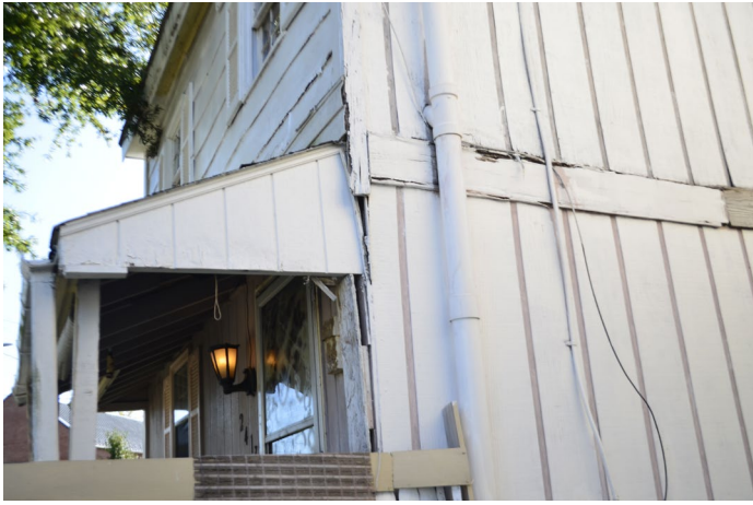
Figure 7. View of the poor condition of the siding and porch roof on the west side of 2417 Carrington Street.
