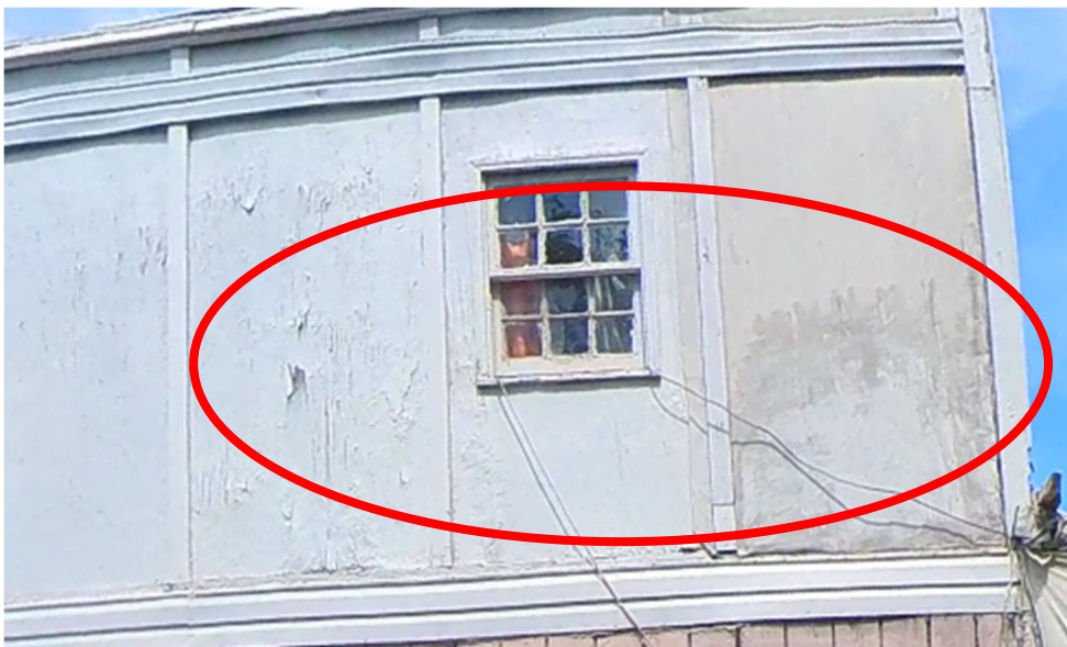
Painted plywood panels were used to sheath the rear of the home. The panels are rotting.
