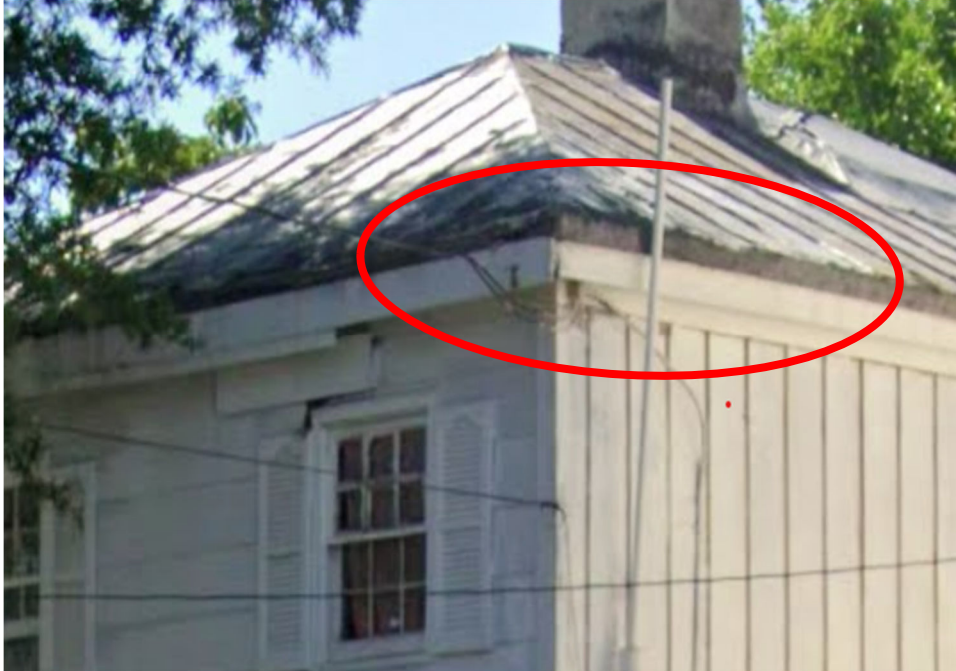
Extensive rot is present in the roof structure.
