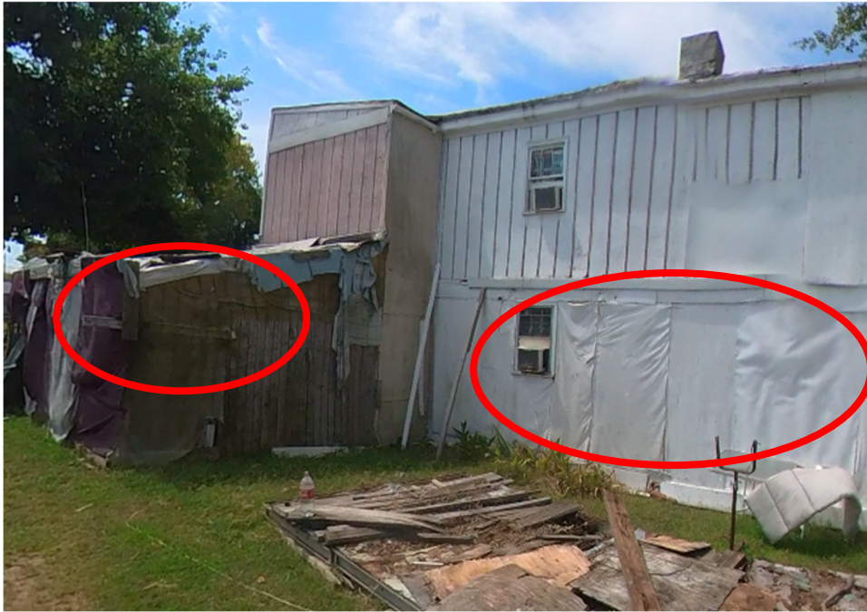
The homes siding was removed and replaced with a mix of materials, all of which has begun to rot.
