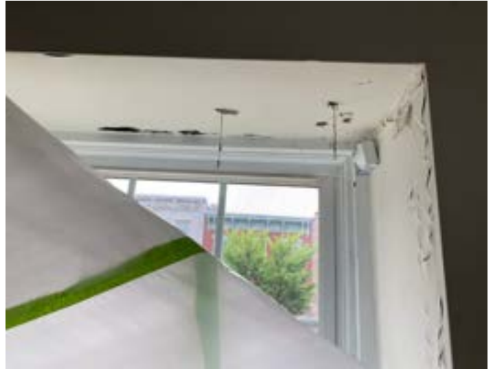
Figure 4. Interior water damage and mold
