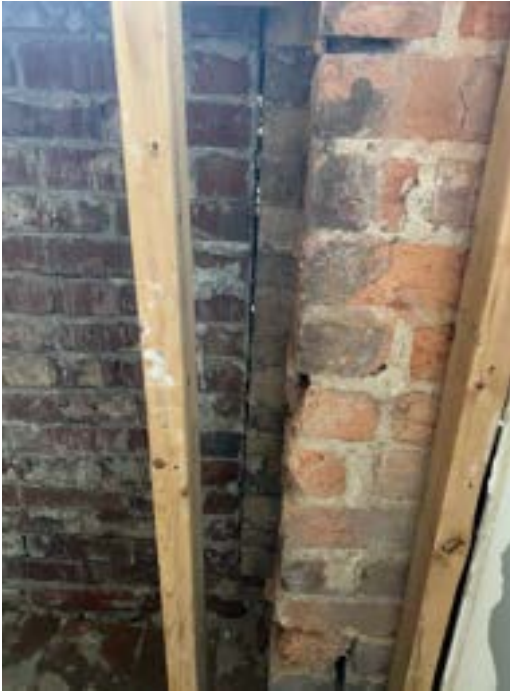
Figure 3. Brick infill separating from original masonry opening. Exposed to outside
