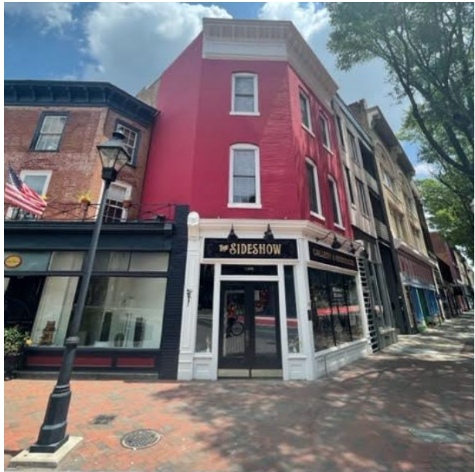
Figure 4. Painted & unpainted masonry on subject block. Brick painted to resemble brick color.
