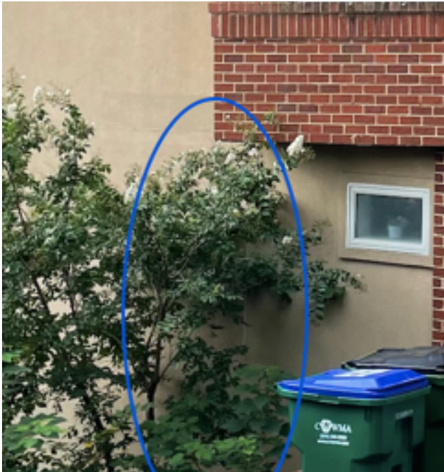
Settling bay location that needs support
