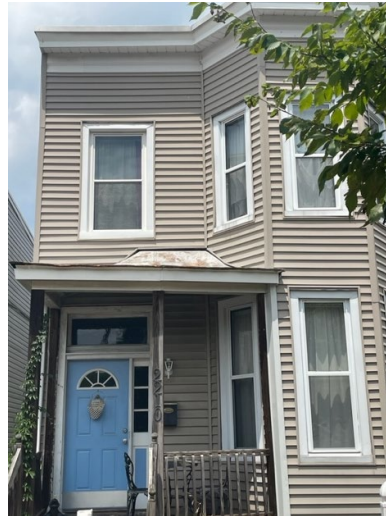
Figure 4. Existing porch roof condition.
