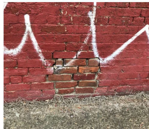
Figure 6. Detail of damaged brick
