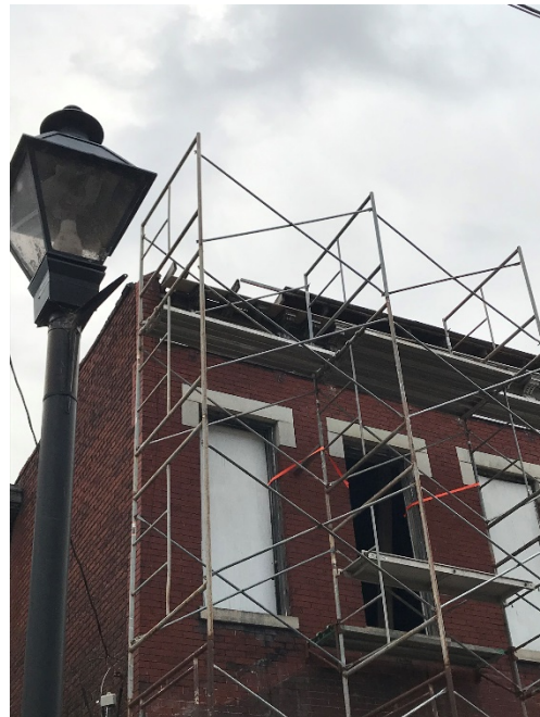
Figure 4. Section of missing cornice.
